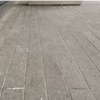
5 Grey granite paving slabs to Business School landscaping
