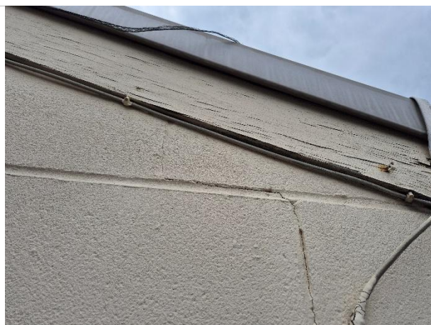
Photo 11: Sealed timber fascia at (north-eastern elevation) to be removed
