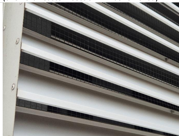
Photo 16: Mesh at louvered air vents
