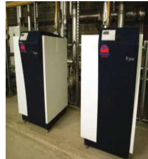
Existing Domestic Hot Water Andrews Water Heater
