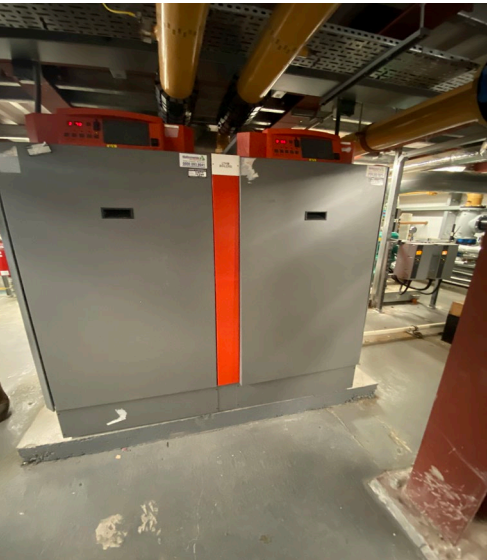
Existing Gas Fired Heating Boilers
