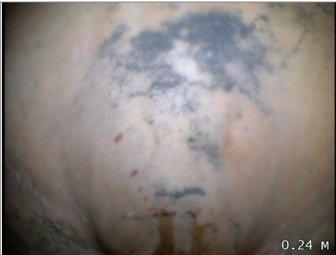
Line of drain/sewer deviates down
