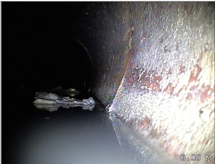
Settled deposits coarse 10% cross-sectional area loss
