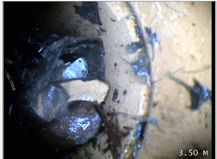
Survey abandoned - Remark: DEBRIS - 80%
