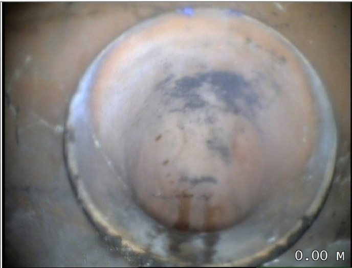
Start node type, gully, reference GULLY 1
