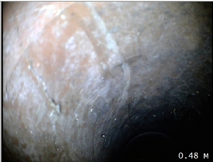
Line of drain/sewer deviates down
