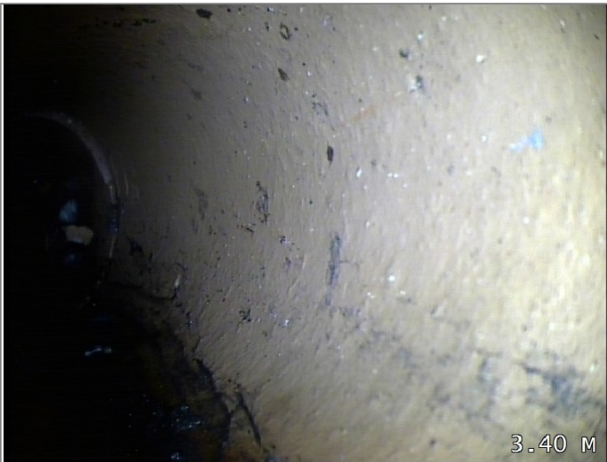
Line of drain/sewer deviates left
