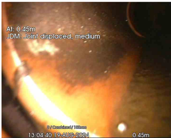
17_0-45m_130440.jpg, 00:00:15, 0.45 m Joint displaced, medium
