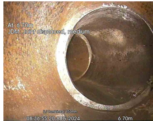
25_6-70m_083655.jpg, 00:00:43, 6.70 m Joint displaced, medium
