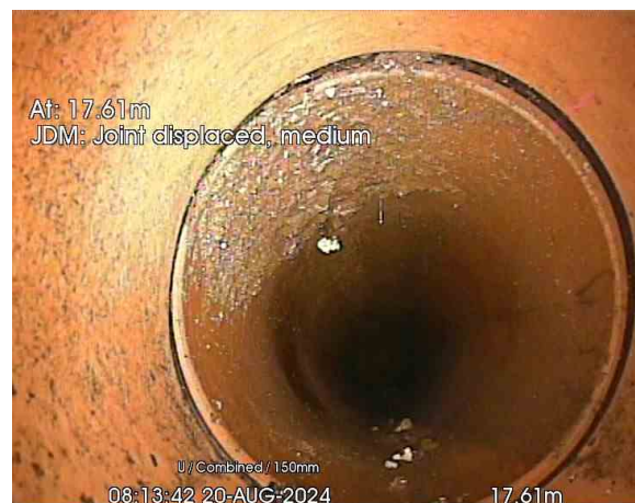
21_17-61m_081342.jpg, 00:02:27, 17.61 m Joint displaced, medium
