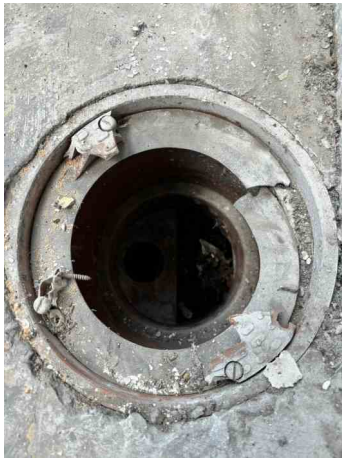
RWP5X_5599972a-860a-463b-8a4b-9bf7521c9f5e_20240905_103716.jpg, 0.00 m General remark, Broken Access Lid Requires Replacement
