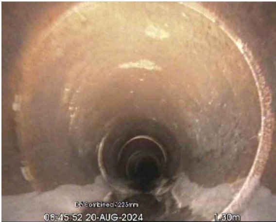
EXMH01X_316b20f6-49c9-47a9-89c7-6b1c2c5e5027_20240820_111157_865.jpg, 00:00:05, 1.30 m Joint displaced, medium
