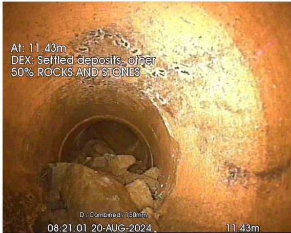
23_11-43m_082101.jpg, 00:01:25, 11.43 m Settled deposits, other, 50% cross-sectional area loss, ROCKS AND STONES
