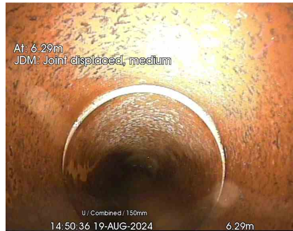
19_6-29m_145036.jpg, 00:01:09, 6.29 m Joint displaced, medium
