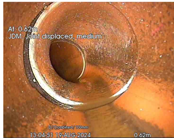
17_0-62m_130451.jpg, 00:00:20, 0.62 m Joint displaced, medium
