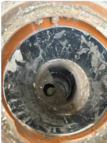
RWP17X_907a7d9f-ff82-4447-b876-72ac78f6b15f_20240905_114840.jpg, 0.00 m General remark, Broken Access Lid Requires Replacement
