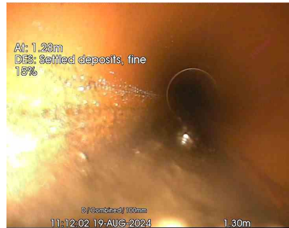
12_1-30m_111202.jpg, 00:00:19, 1.30 m Settled deposits, fine, 15% cross-sectional area loss
