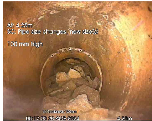
22_4-25m_081700.jpg, 00:00:41, 4.25 m Pipe size changes, new size(s), 100mm high
