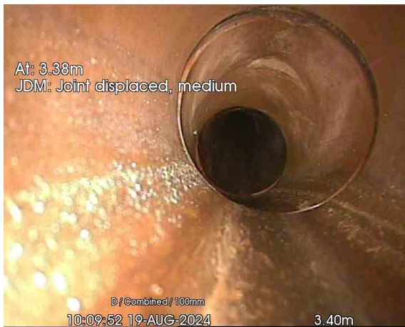
At: 3.38m JDM: Joint displaced, medium D:/Combined/100mm 10:09:52 19-AUG-2024 3.40m 4_3-43m_100952.jpg, 00:00:29, 3.43 m Joint displaced, medium
