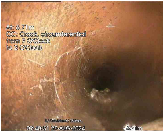
28_6-71m_094051.jpg, 00:01:03, 6.71 m Crack, circumferential from 7 o'clock to 2 o'clock
