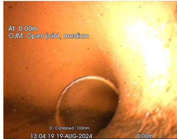
17_0-00m_130419.jpg, 00:00:05, 0.00 m Open joint, medium
