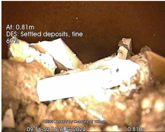
1_0-81m_091653.jpg, 00:00:33, 0.81 m Settled deposits, fine, 60% cross-sectional area loss
