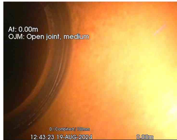
At: 0.00m OJM: Open joint, medium D//Combined/ 100mm 12:43:23 19-AUG-2024 0.00m 14_0-00m_124323.jpg, 00:00:07, 0.00 m Open joint, medium
