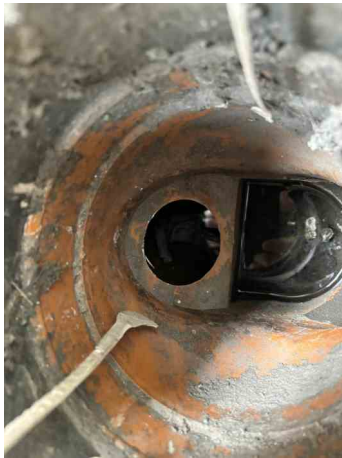
RWP6X_27b0f978-2436-42f0-810a-20b1eb942aa4_20240905_114227.jpg, 0.00 m General remark, Broken Access Lid Requires Replacement
