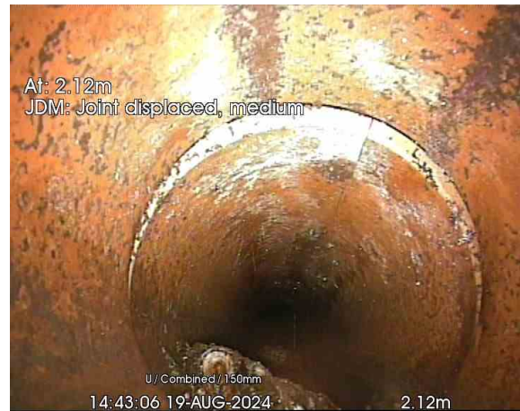
18_2-12m_144306.jpg, 00:00:17, 2.12 m Joint displaced, medium
