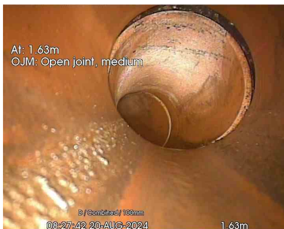
24_1-63m_082742.jpg, 00:00:16, 1.63 m Open joint, medium
