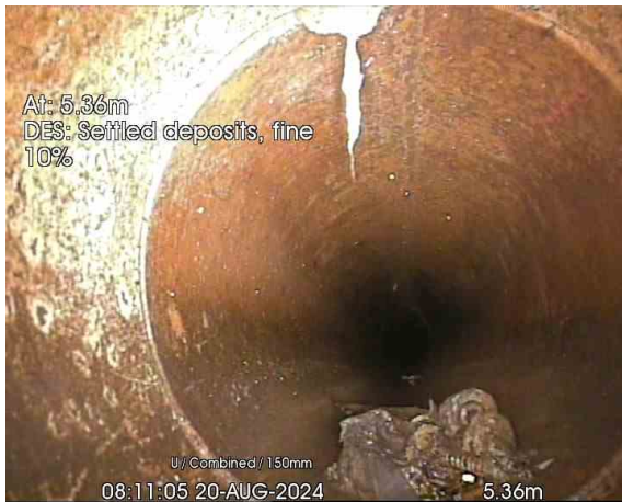
21_5-36m_081105.jpg, 00:00:39, 5.36 m Settled deposits, fine, 10% cross-sectional area loss
