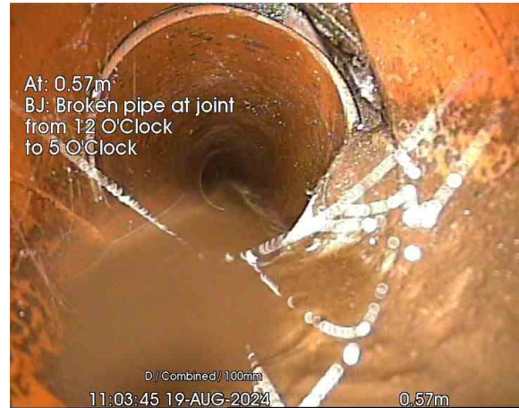
9_0-57m_110345.jpg, 00:00:20, 0.57 m Broken pipe at joint from 12 o'clock to 5 o'clock
