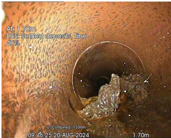
29_1-70m_094625.jpg, 00:00:15, 1.70 m Settled deposits, fine, 40% cross-sectional area loss
