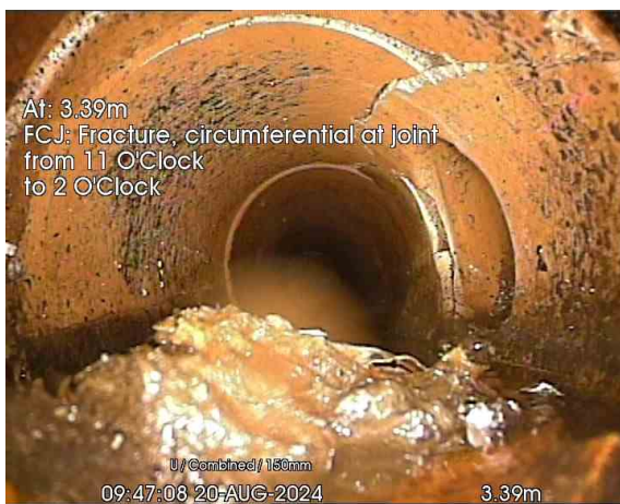
29_3-39m_094708.jpg, 00:00:41, 3.39 m Fracture, circumferential at joint from 11 o'clock to 2 o'clock
