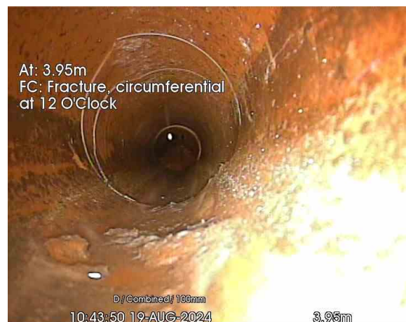
7_3-95m_104350.jpg, 00:00:48, 3.95 m Fracture, circumferential at 12 o'clock
