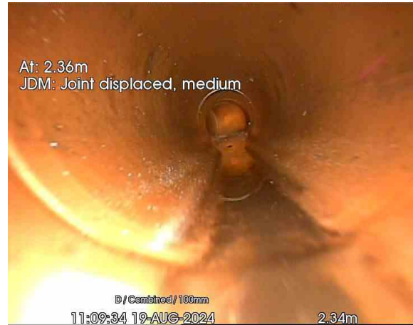
11_2-29m_110934.jpg, 00:00:26, 2.29 m Joint displaced, medium
