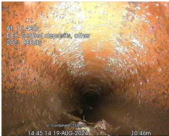
18_10-46m_144514.jpg, 00:01:24, 10.46 m Settled deposits, other, 20% cross-sectional area loss, DEBRIS
