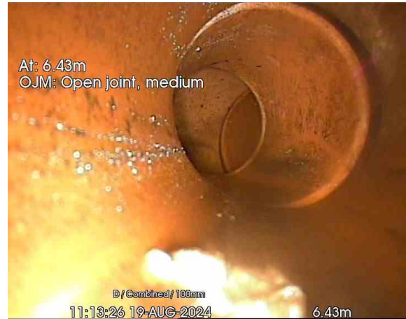
12_6-43m_111326.jpg, 00:01:18, 6.43 m Open joint, medium
