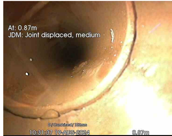
5_0-87m_103137.jpg, 00:00:16, 0.87 m Joint displaced, medium
