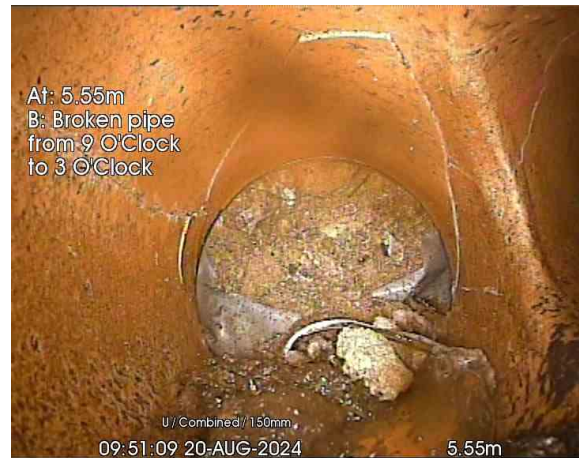
29_5-55m_095109.jpg, 00:02:43, 5.55 m Broken pipe from 9 o'clock to 3 o'clock
