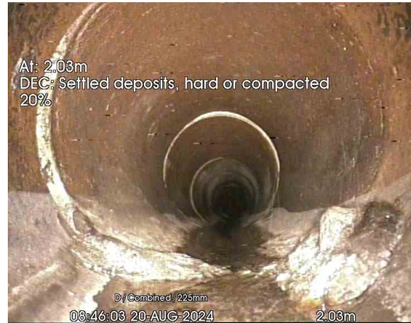
27_2-03m_084603.jpg, 00:00:08, 2.03 m Settled deposits, hard or compacted, 20% cross-sectional area loss
