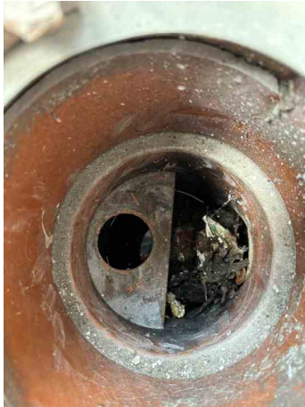
RWP13X_91cde4ee-e51f-48cb-b6a5-6c27560fd97b_20240905_113519.jpg, 0.00 m General remark, Broken Access Cover Needs Replacement
