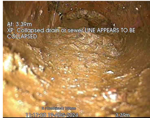
13_3-39m_111700.jpg, 00:00:51, 3.39 m Collapsed drain or sewer, LINE APPEARS TO BE COLLAPSED
