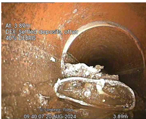
28_3-89m_094007.jpg, 00:00:38, 3.89 m Settled deposits, other, 40% cross-sectional area loss, DEBRIS
