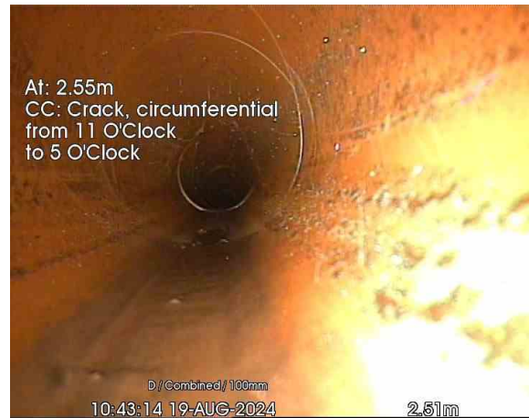
7_2-51m_104314.jpg, 00:00:27, 2.51 m Crack, circumferential from 11 o'clock to 5 o'clock
