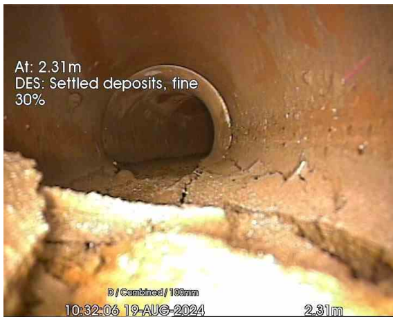
5_2-31m_103206.jpg, 00:00:29, 2.31 m Settled deposits, fine, 30% cross-sectional area loss
