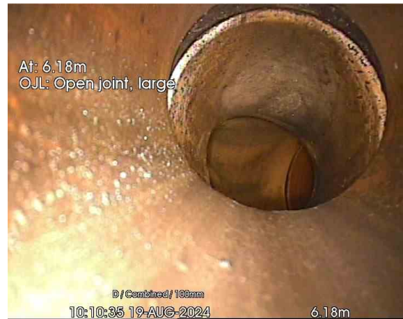
4_6-18m_101035.jpg, 00:00:52, 6.18 m Open joint, large
