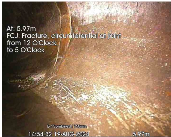
20_5-97m_145432.jpg, 00:00:59, 5.97 m Fracture, circumferential at joint from 12 o'clock to 5 o'clock
