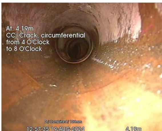
16_4-19m_125735.jpg, 00:00:49, 4.19 m Crack, circumferential from 4 o'clock to 8 o'clock
