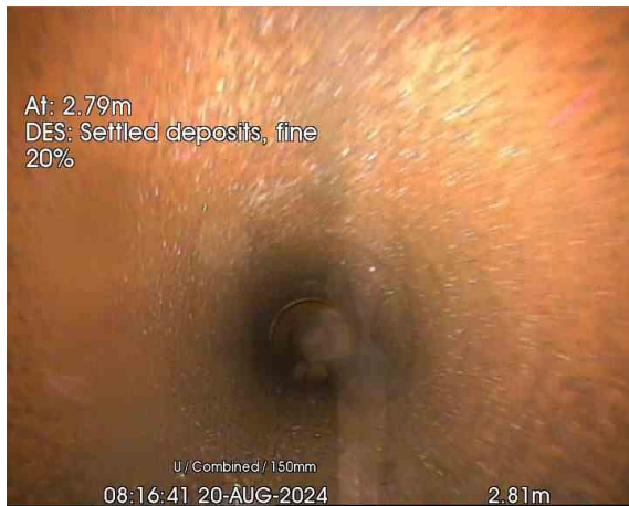
22_2-81m_081641.jpg, 00:00:28, 2.81 m Settled deposits, fine, 20% cross-sectional area loss
