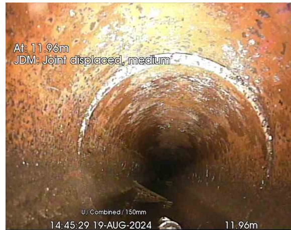
18_11-96m_144529.jpg, 00:01:35, 11.96 m Joint displaced, medium
