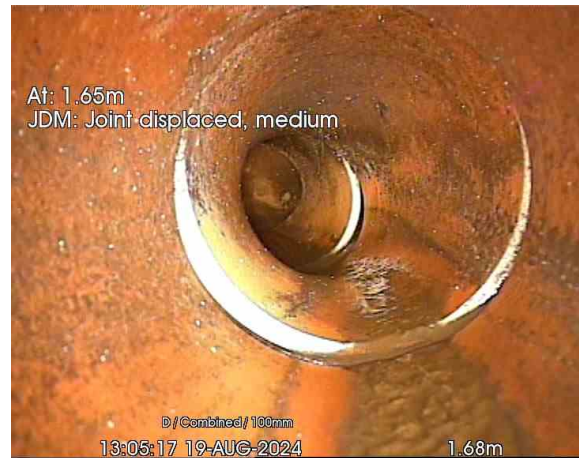
17_1-68m_130517.jpg, 00:00:33, 1.68 m Joint displaced, medium
