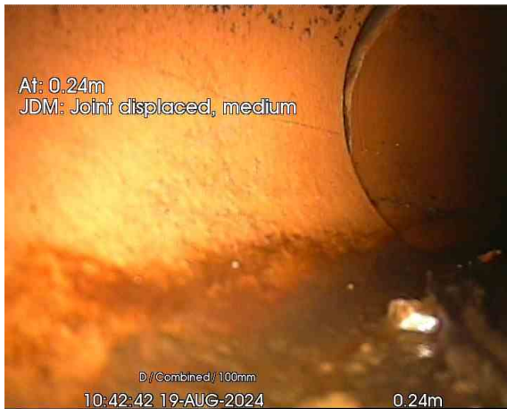
7_0-24m_104242.jpg, 00:00:06, 0.24 m Joint displaced, medium
