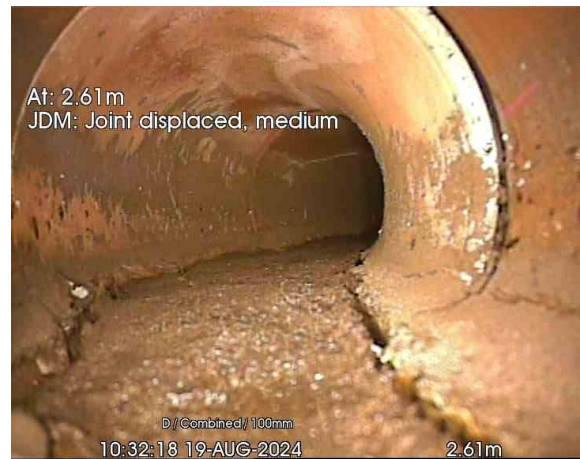
5_2-61m_103218.jpg, 00:00:35, 2.61 m Joint displaced, medium
