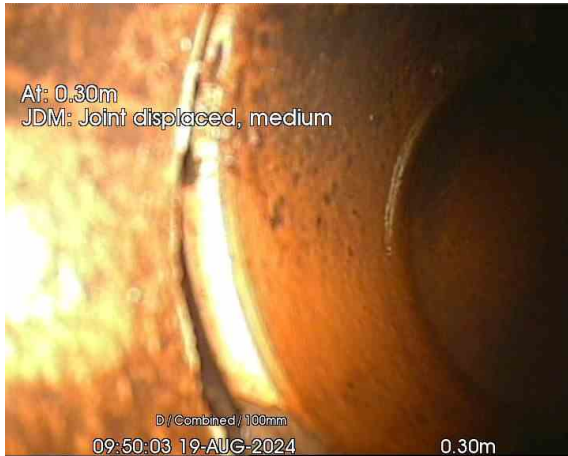
3_0-30m_095003.jpg, 00:00:14, 0.30 m Joint displaced, medium
