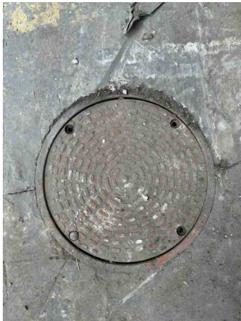
RWP14X_2ad96ba6-5eff-4e72-90f0-200b78f6413f_20240905_113532.jpg, 0.00 m General remark, Broken Access Cover Needs Replacement
