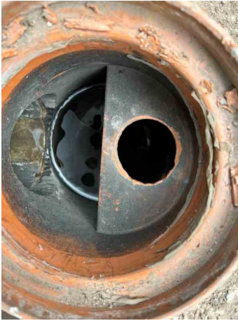
RWP7X_a4eca916-7136-412f-b775-93861f9280f0_20240905_114853.jpg, 0.00 m General remark, Broken Access Lid Requires Replacement
