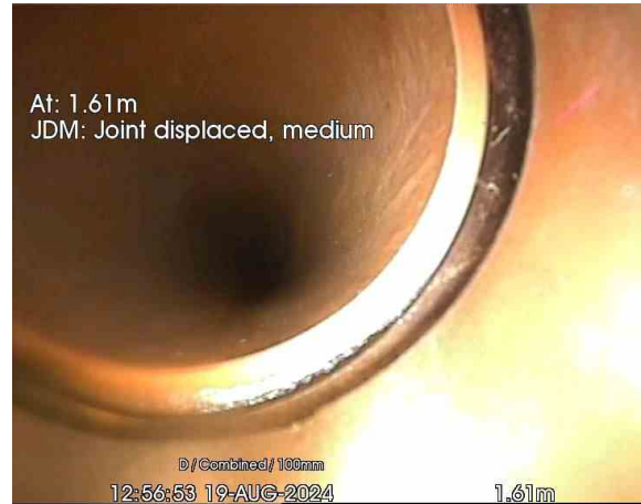
16_1-61m_125653.jpg, 00:00:18, 1.61 m Joint displaced, medium
