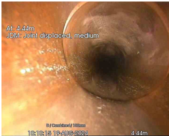
4_4-44m_101015.jpg, 00:00:41, 4.44 m Joint displaced, medium
