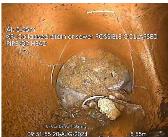
29_5-55m_095155.jpg, 00:02:50, 5.55 m Collapsed drain or sewer, 95% cross-sectional area loss, COLLAPSED PIPE
