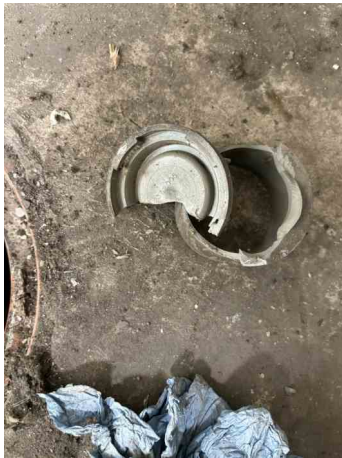
RWP16X_c5d723e4-e0a0-48a6-a805-8d378c865f74_20240905_114107.jpg, 0.00 m General remark, Broken Access Lid Requires Replacement
