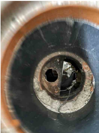
RWP8X_ad5343f8-cd06-4858-a02e-798d3058c832_2024090 5_113446.jpg, 0.00 m General remark, Broken Access Cover Needs Replacement
