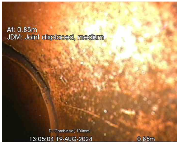
17_0-85m_130504.jpg, 00:00:26, 0.85 m Joint displaced, medium
