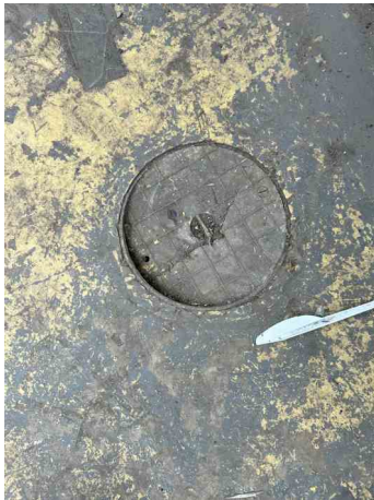
RWP15X_f2e56978-4e56-48f7-bcb2-de8d70743969_20240905_115028.jpg, 0.00 m General remark, Broken Access Lid Requires Replacement
