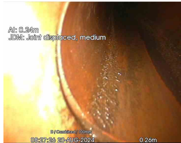
24_0-28m_082726.jpg, 00:00:06, 0.28 m Joint displaced, medium
