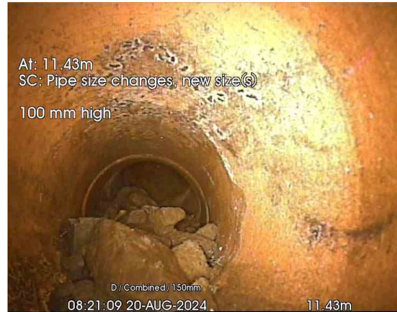
23_11-43m_082109.jpg, 00:01:28, 11.43 m Pipe size changes, new size(s), 100mm high
