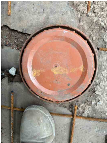
RWP10X_5029c86c-830b-4f51-9694-0b2e8bad07b9_20240905_113458.jpg, 0.00 m General remark, Broken Access Cover Needs Replacement
