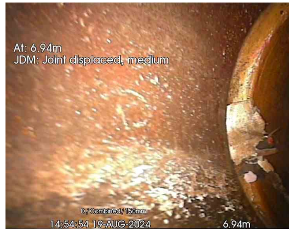
20_6-94m_145454.jpg, 00:01:10, 6.94 m Joint displaced, medium
