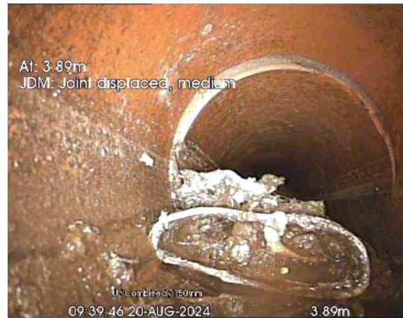
RE04X_7c4d29cc-008c-4ad1-8582-84f3936c5463_20240820_111352_621.jpg, 00:00:34, 3.89 m Joint displaced, medium
