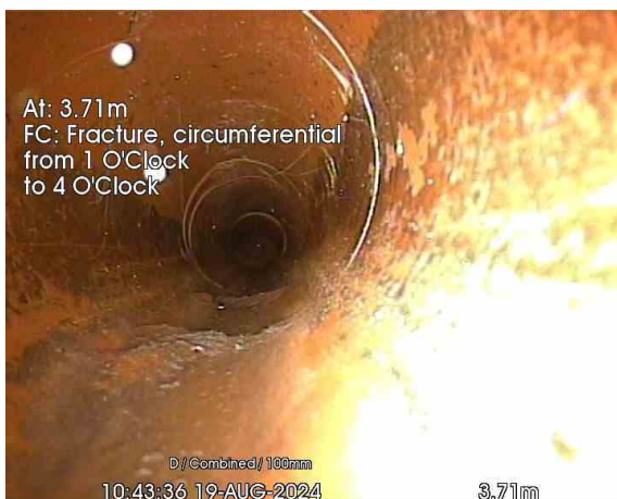
7_3-71m_104336.jpg, 00:00:40, 3.71 m Fracture, circumferential from 1 o'clock to 4 o'clock
