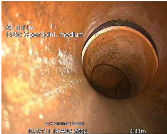
6_4-41m_103711.jpg, 00:00:56, 4.41 m Open joint, medium
