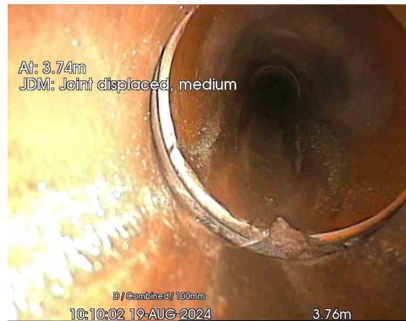
At: 3.74m JDM: Joint displaced, medium D:/Combined/100mm 10:10:02 19-AUG-2024 3.76m 4_3-76m_101002.jpg, 00:00:34, 3.76 m Joint displaced, medium
