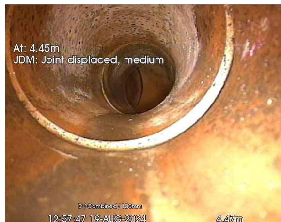
16_4-47m_125747.jpg, 00:00:55, 4.47 m Joint displaced, medium
