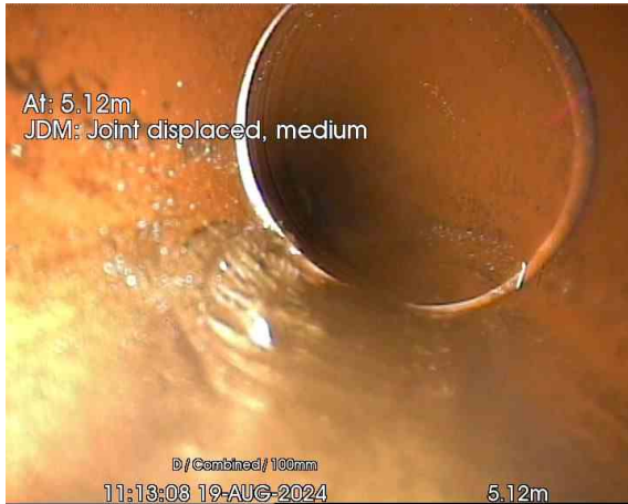
12_5-12m_111308.jpg, 00:01:06, 5.12 m Joint displaced, medium
