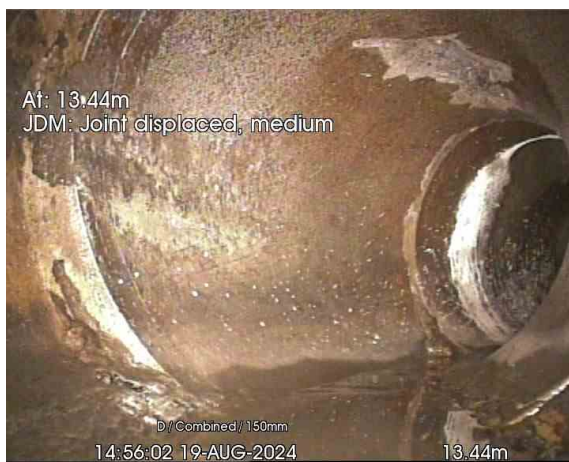
20_13-44m_145602.jpg, 00:01:52, 13.44 m Joint displaced, medium
