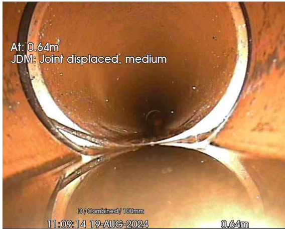
11_0-64m_110914.jpg, 00:00:13, 0.64 m Joint displaced, medium
