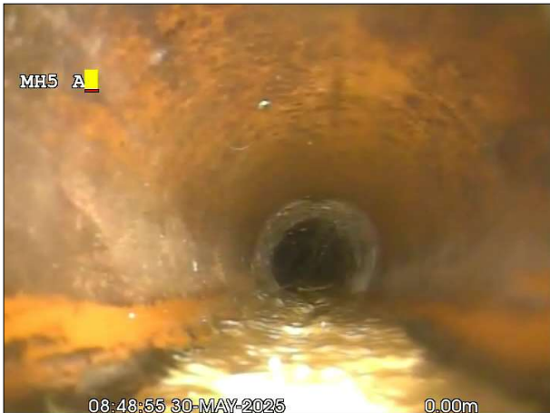
Photo: 58_4a, 00:00:00 0.1m, Debris grease, from 05 to 07 o'clock, 5 % cross-sectional area loss
