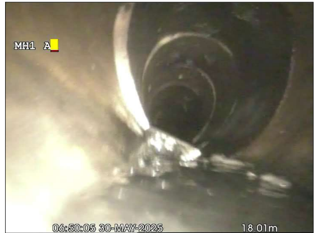
Photo: 1_12b, 00:00:00 17.5m, Joint displaced. Medium
