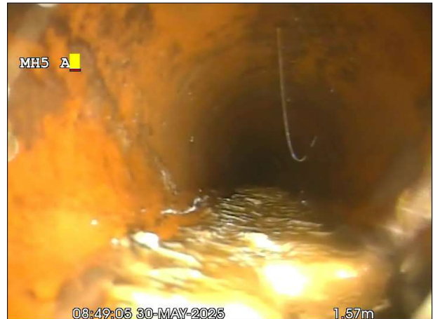
Photo: 59_5a, 00:00:00 1.6m, Debris grease, from 05 to 07 o'clock, 10 % cross-sectional area loss
