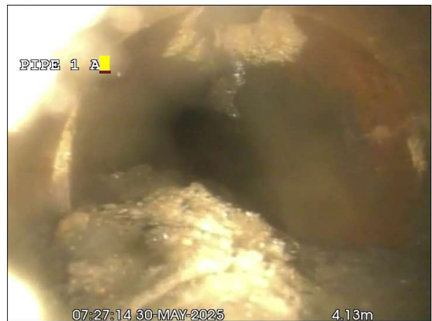
Photo: 9_14a, 00:00:00 4.1m, Debris, 40 % cross-sectional area loss
