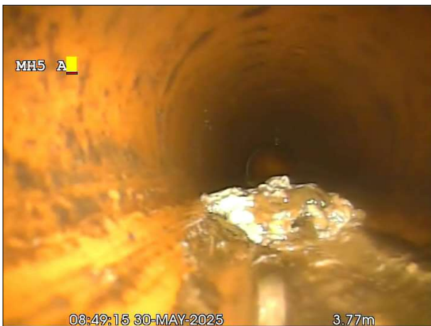
Photo: 60_6a, 00:00:00 4m, Debris grease, from 04 to 08 o'clock, 20 % cross-sectional area loss
