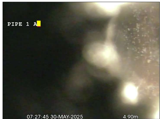
Photo: 9_17a, 00:00:00 4.9m, Survey abandoned, Remark: Unable to survey beyond this point due to blockage.
