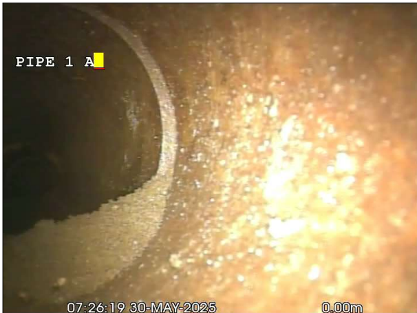
Photo: 82_4a, 00:00:00 0.2m, Debris, 20 % cross-sectional area loss
