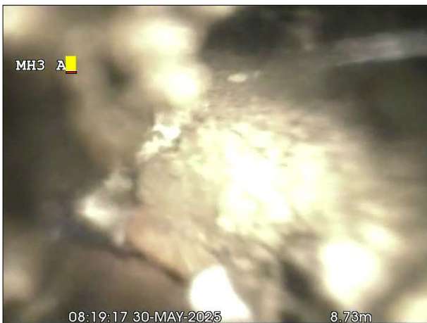
Photo: 32_12a, 00:00:00 8.8m, Survey abandoned, Remark: Unable to survey beyond this point due to blockage.
