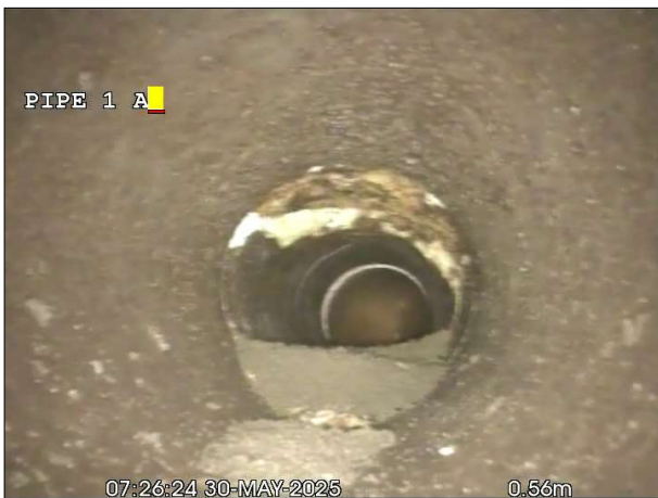
Photo: 9_6a, 00:00:00 0.7m, Debris, 40 % cross-sectional area loss
