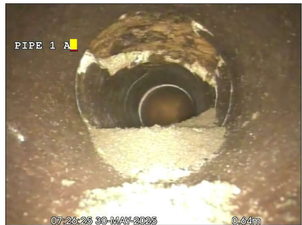
Photo: 9_7a, 00:00:00 0.8m, Surface damage, spalling large, from 10 to 02 o'clock
