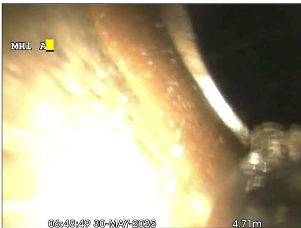
Photo: 6_6a, 00:00:00 4.8m, Joint displaced. Medium
