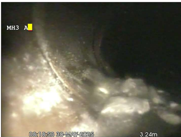
Photo: 26_6a, 00:00:00 3.3m, Debris, 10 % cross-sectional area loss
