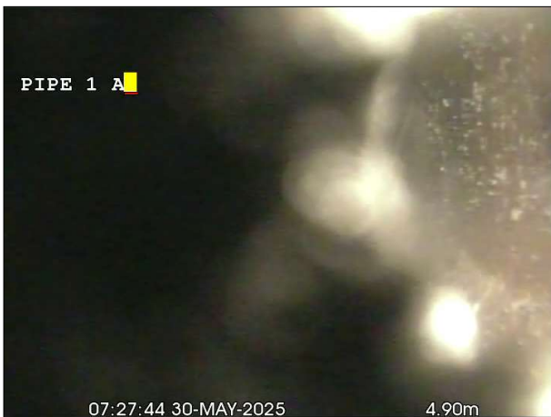
Photo: 9_16a, 00:00:00 4.9m, Debris, 95 % cross-sectional area loss
