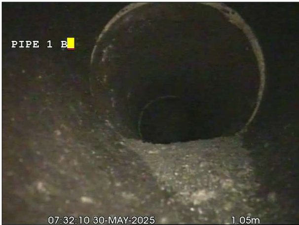
Photo: 100_5a, 00:00:00 1.1m, Debris, 10 % cross-sectional area loss
