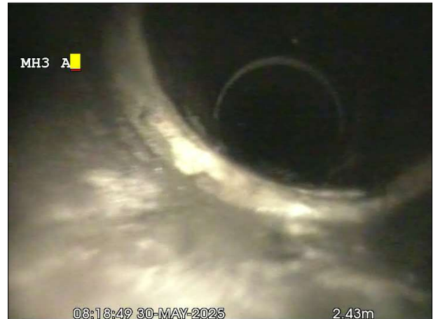
Photo: 25_5a, 00:00:00 2.5m, Joint displaced. Medium
