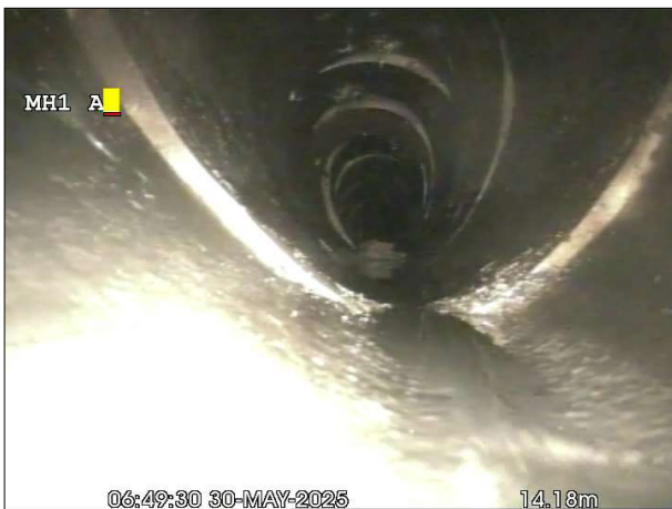
Photo: 11_10a, 00:00:00 14.3m, Joint displaced. Medium
