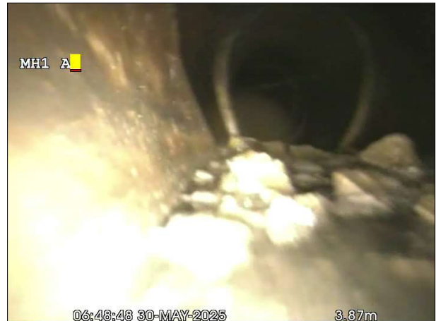
Photo: 5_5a, 00:00:00 3.9m, Debris, 10 % cross-sectional area loss
