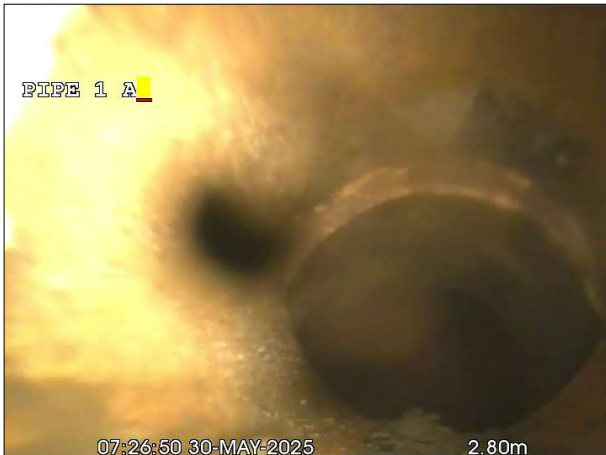
Photo: 9_9a, 00:00:00 2.9m, Joint displaced. Large
