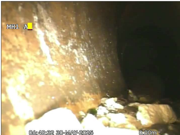
Photo: 4_4a, 00:00:00 0.05m, Debris, 5 % cross-sectional area loss
