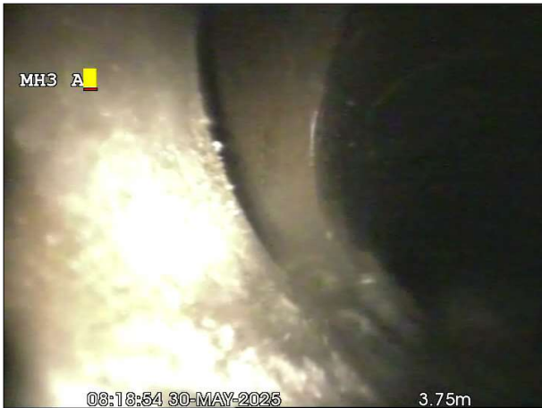
Photo: 27_7b, 00:00:00 3.7m, Junction at 09 o'clock, dia 150 mm
