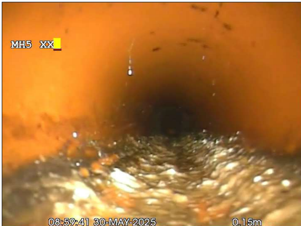
Photo: 74_4a, 00:00:00 0.1m, Debris grease, from 05 to 07 o'clock, 5 % cross-sectional area loss
