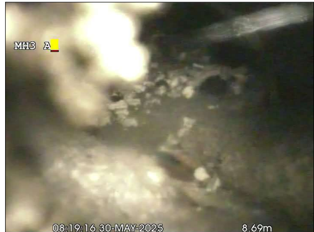
Photo: 31_11b, 00:00:00 8.8m, Debris, 95 % cross-sectional area loss
