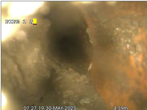
Photo: 9_15a, 00:00:00 4.4m, Debris, 80 % cross-sectional area loss
