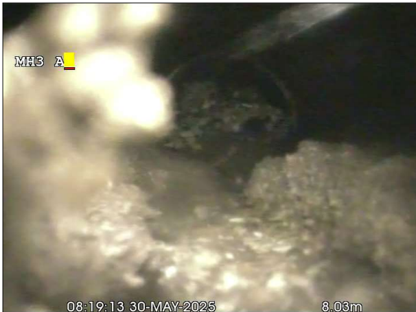
Photo: 31_11a, 00:00:00 8.8m, Debris, 95 % cross-sectional area loss
