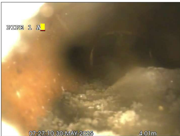
Photo: 9_13a, 00:00:00 4m, Debris, 30 % cross-sectional area loss
