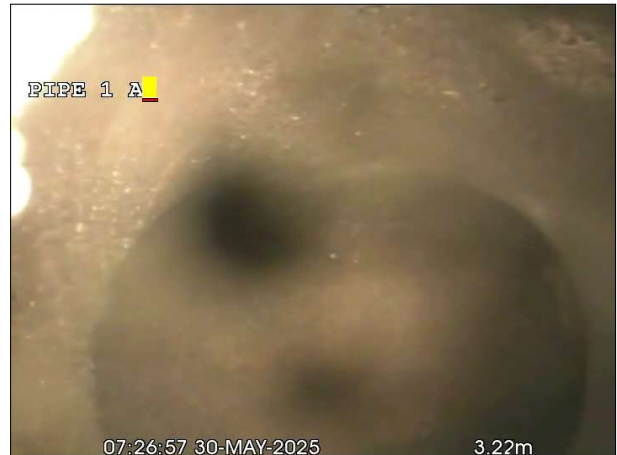
Photo: 9_11a, 00:00:00 3.5m, General Observation, Remark: Drops into sewer line.
