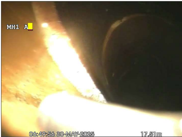
Photo: 1_12a, 00:00:00 17.5m, Joint displaced. Medium
