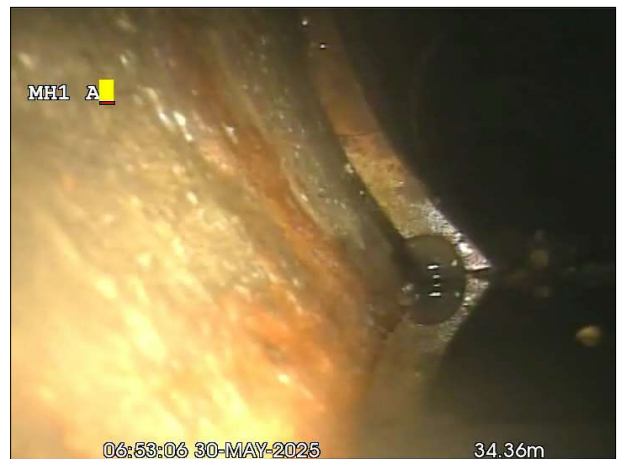
Photo: 1_17a, 00:00:00 34.5m, Joint displaced. Medium
