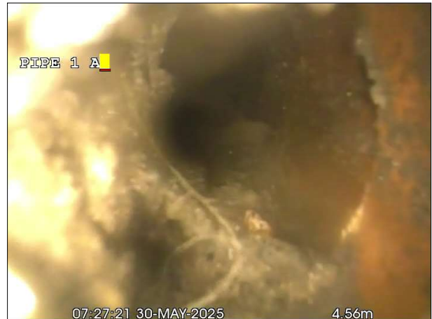
Photo: 9_15b, 00:00:00 4.4m, Debris, 80 % cross-sectional area loss
