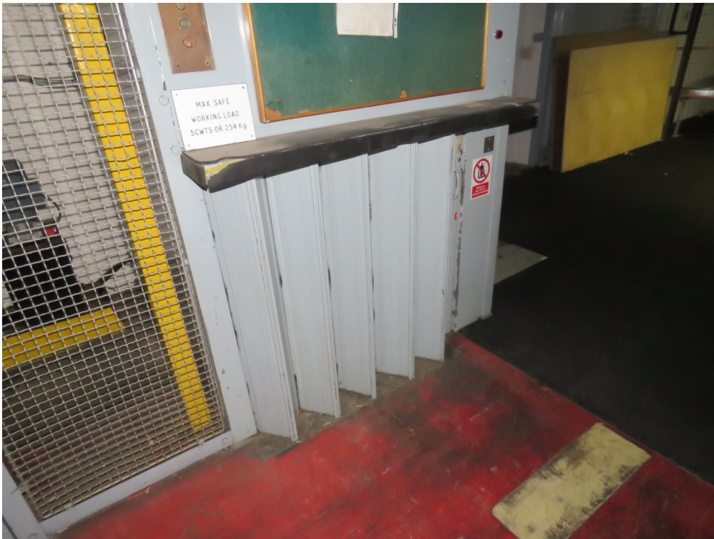
B-27 Non-passenger lift between basement levels.
