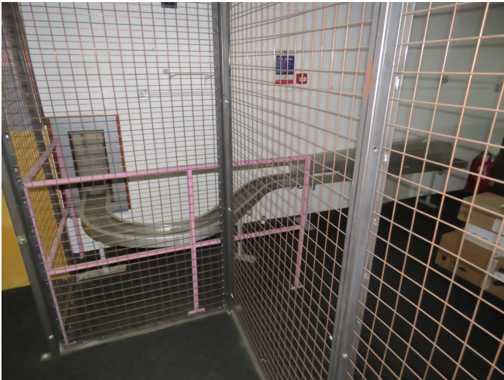
B1-23 View of the Telelift within the document store.
