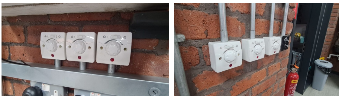
Image 5: 2x control panels for the fans allowing inflow and extraction for air exchange
