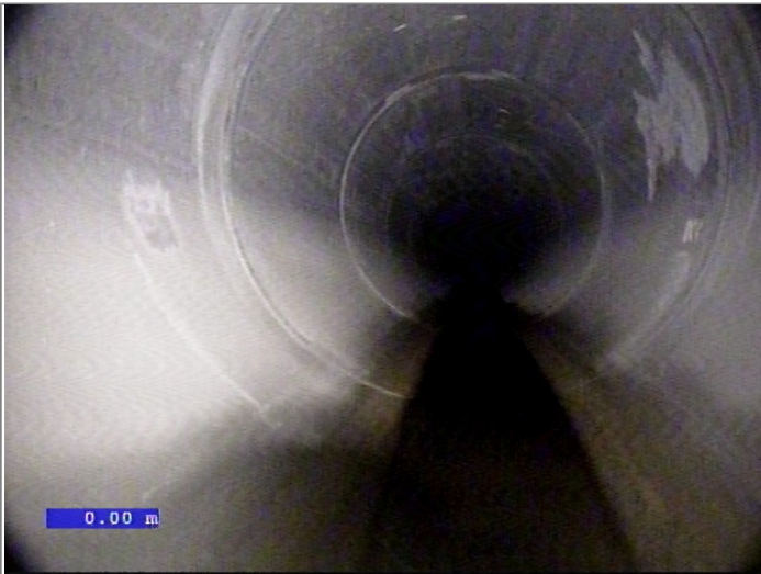
Start node type, manhole, reference S102
