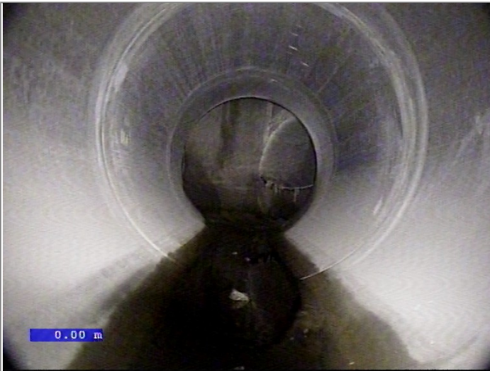
Start node type, manhole, reference S103
