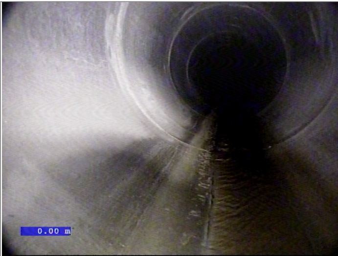
Start node type, manhole, reference S104
