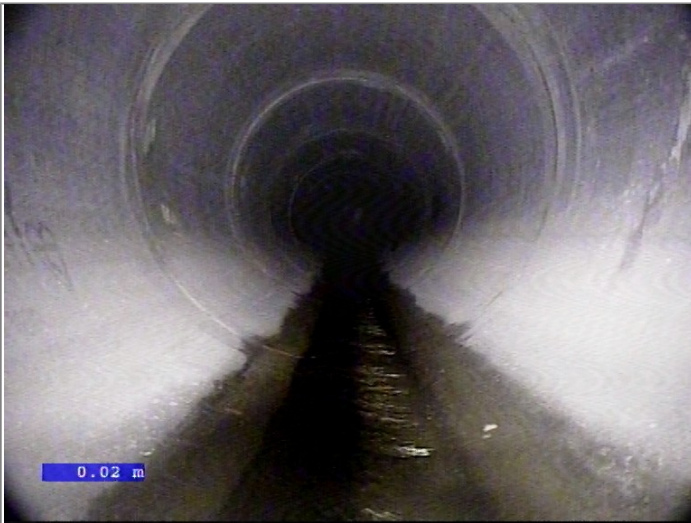
Start node type, manhole, reference S105
