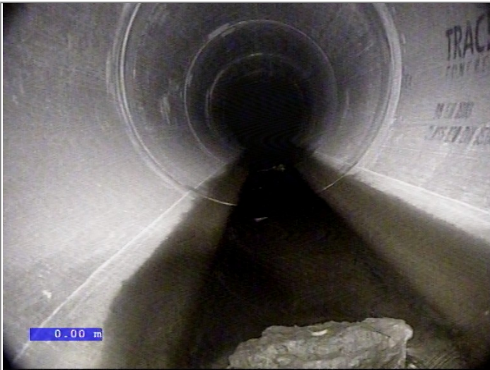
Start node type, manhole, reference S101
