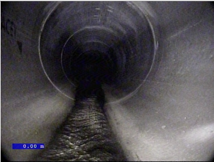
Start node type, manhole, reference S106
