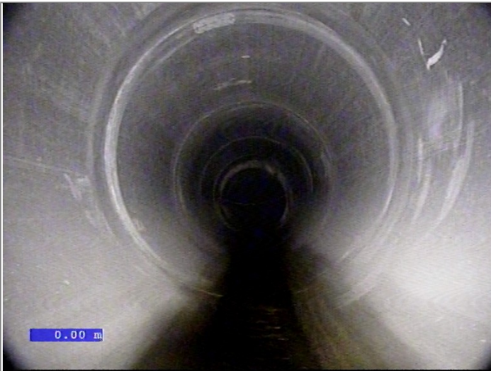
Start node type, manhole, reference S101
