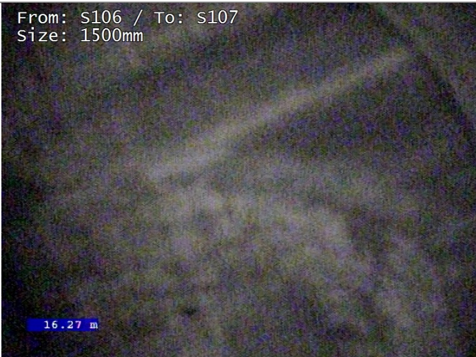
Survey abandoned - Remark: CCTV UNABLE TOMPSS 15% SILT. CLEANING REQUIRED
