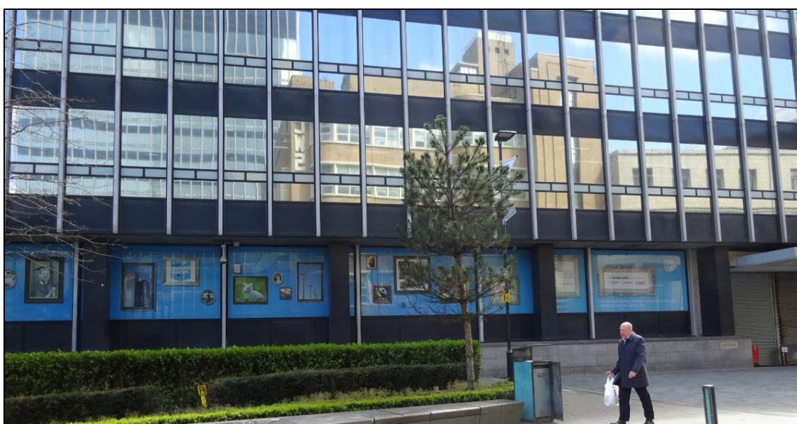
Figure 24. View of the Dantzic Street elevation (2019). The application of the protective film has diminished the intended transparency of the elevations, creating an almost mirror surface.
