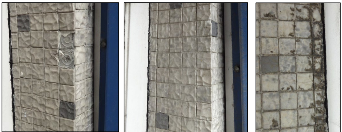
Figure 26. An exposed section of tiling at podium level, showing the pattern of cream and grey blue tiles, as well as the deterioration and discolouration of the surface resulting from atmospheric pollution.
