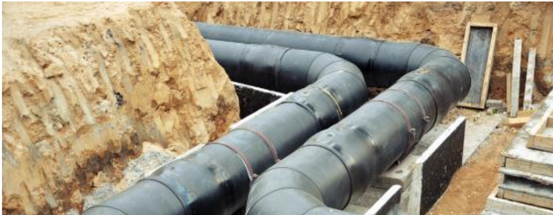
Figure 6.1: Image of District Heating Network Pipework
