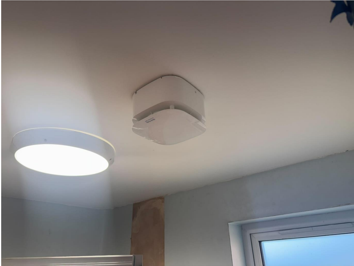
Picture 3 Ventilation Unit
