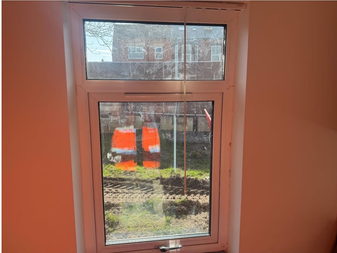
Picture 1 Glazing shown as installed correctly with trickle vents
