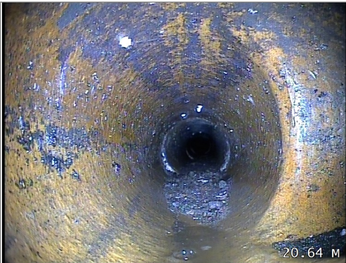
Junction at 3 o'clock, diameter 100mm
