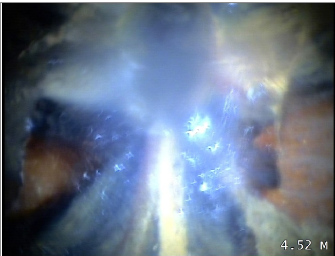
Line of drain/sewer deviates down
