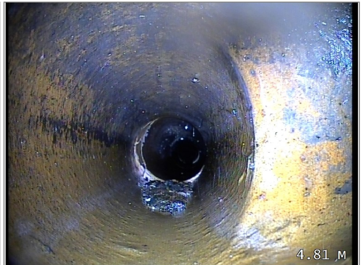
Junction at 3 o'clock, diameter 100mm
