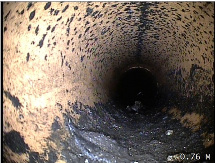
Settled deposits fine 10% cross-sectional area loss
