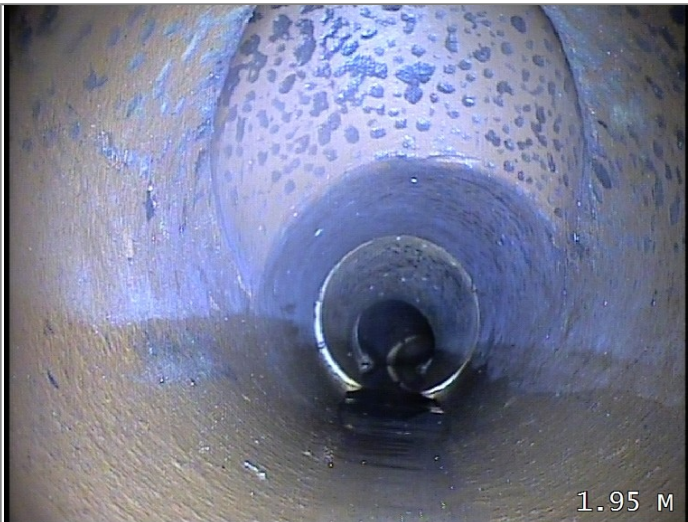
Junction at 12 o'clock, diameter 100mm
