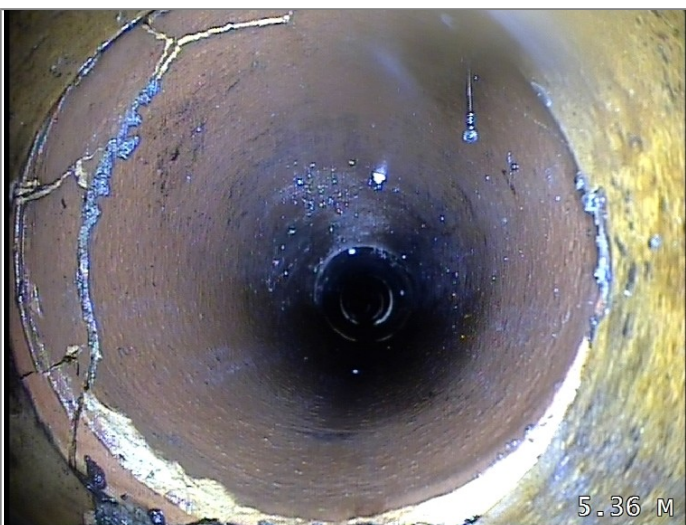
Fracture circumferential from 8 to 12 o'clock
