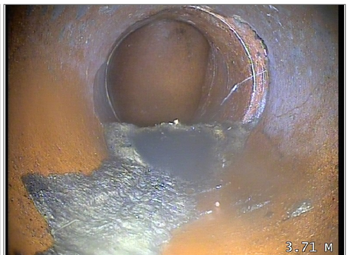
Junction at 12 o'clock, diameter 100mm
