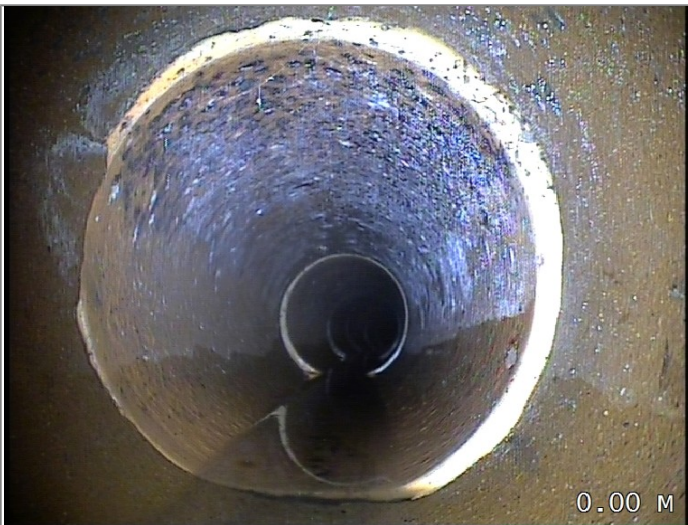
Start node type, manhole, reference INTERNAL MH
