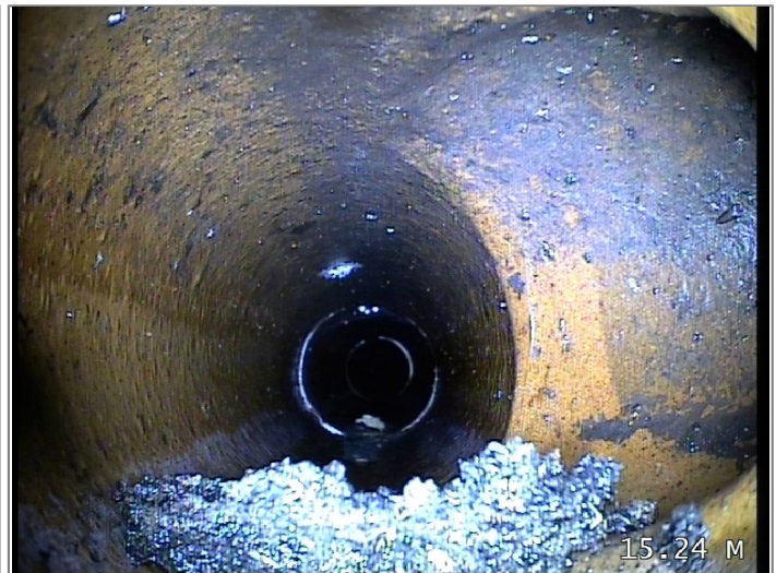
Junction at 3 o'clock, diameter 100mm
