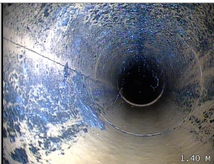
Crack circumferential from 2 to 9 o'clock
