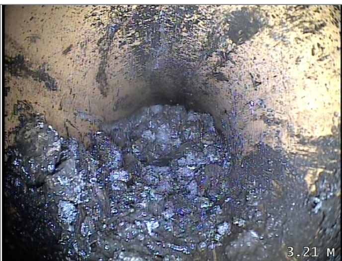
Survey abandoned - Remark: DEBRIS 75%
