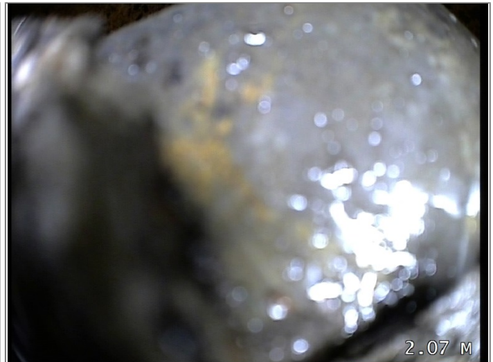
Settled deposits coarse 40% cross-sectional area loss
