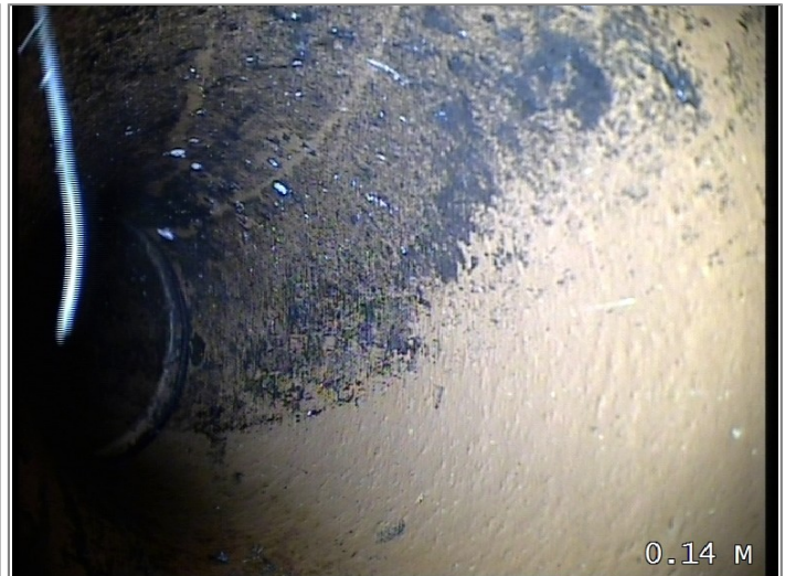
Line of drain/sewer deviates left
