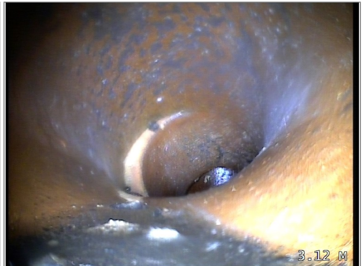
Joint displaced medium
