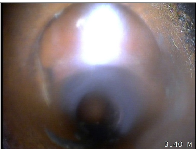
Line of drain/sewer deviates down
