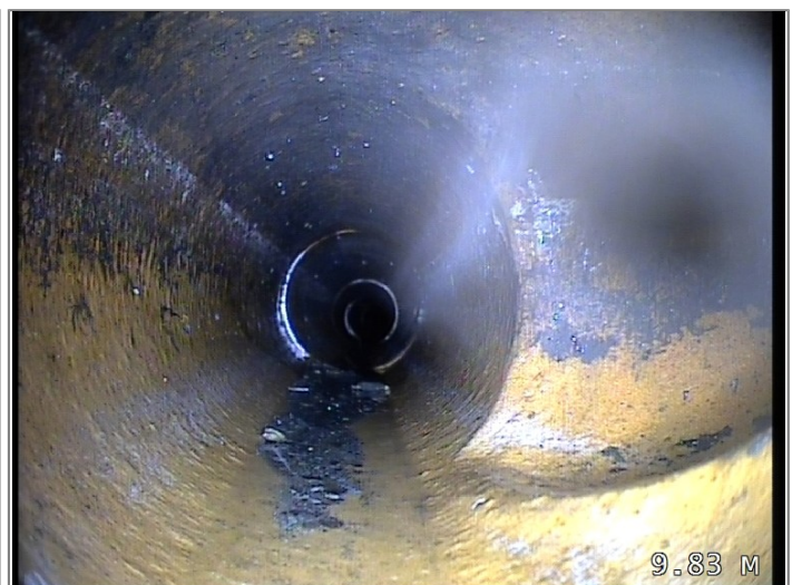
Junction at 3 o'clock, diameter 100mm
