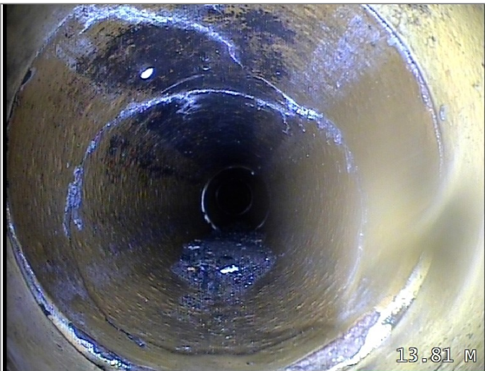
Crack circumferential from 8 to 3 o'clock
