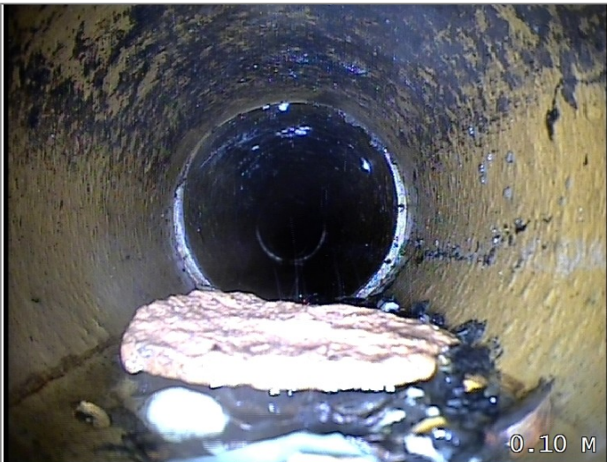
Settled deposits coarse 20% cross-sectional area loss
