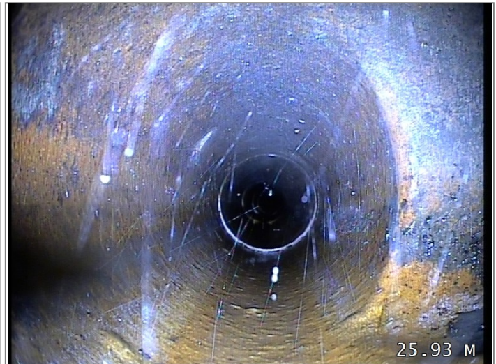
Junction at 3 o'clock, diameter 100mm
