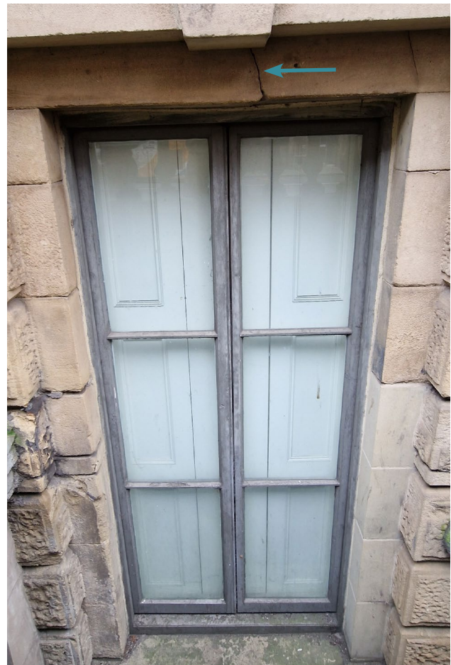
Figure 4 WIN-010 with failed lintel highlighted
