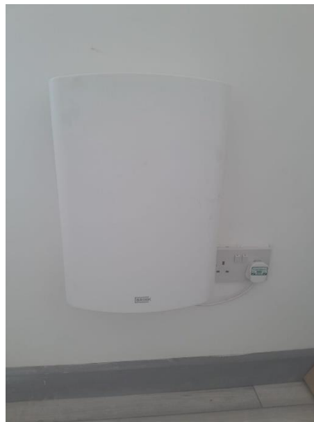
Figure 3 Titon Sonair 3 mechanical ventilation unit, installed at 528 – 532 Hyde Road
