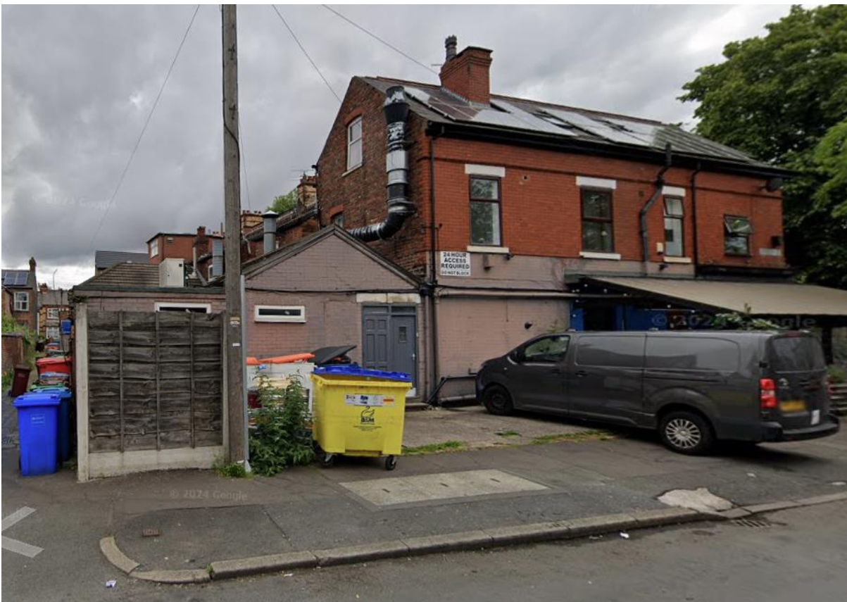
Figure 2 – Extract systems installed at the rear premises of Manchester Road.
