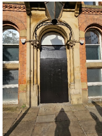
Photograph 6: Boarded entrance to basement floor
