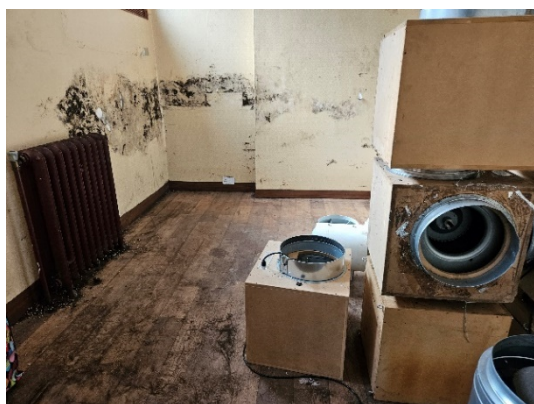
Photograph 11: Derelict room within basement level
