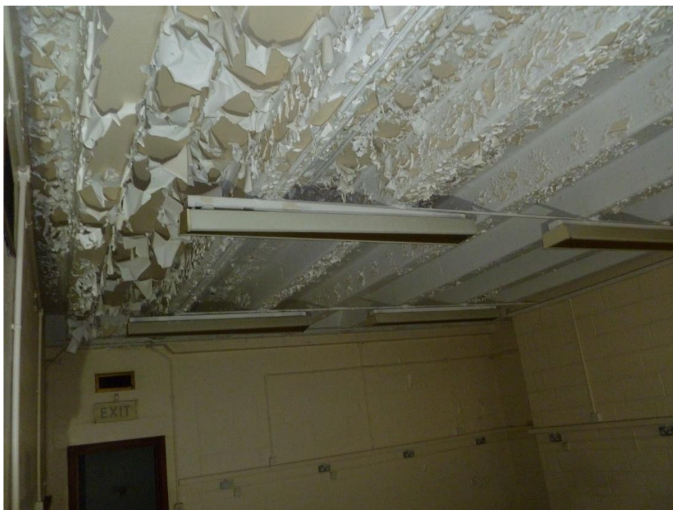
Figure 6.3: Deterioration of paint finishes to ceilings, likely due to damp/water ingress.
