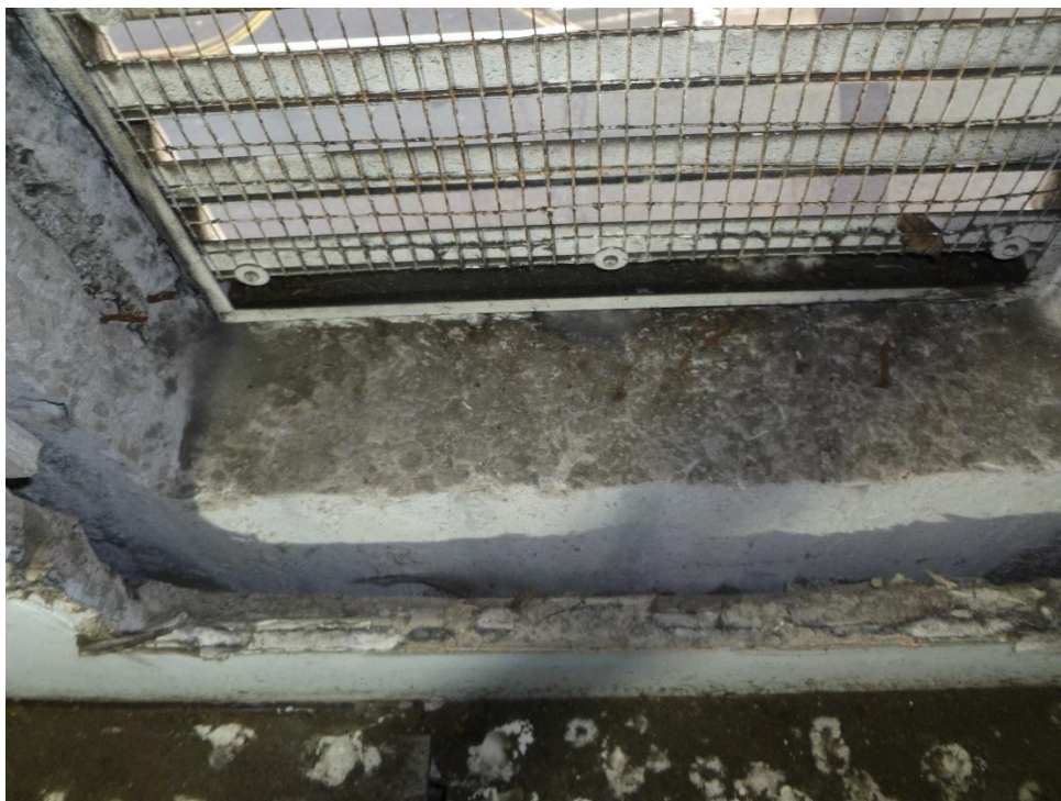
Figure 6.5: View through the building façade where a vent has been inserted revealing the building construction is without insulation.
