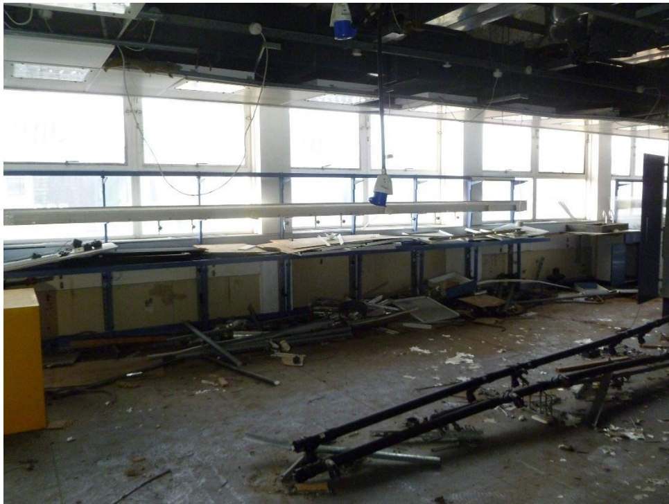
Figure 6.4: Metal theft has resulted in extensive damage to some of the lower floors.
