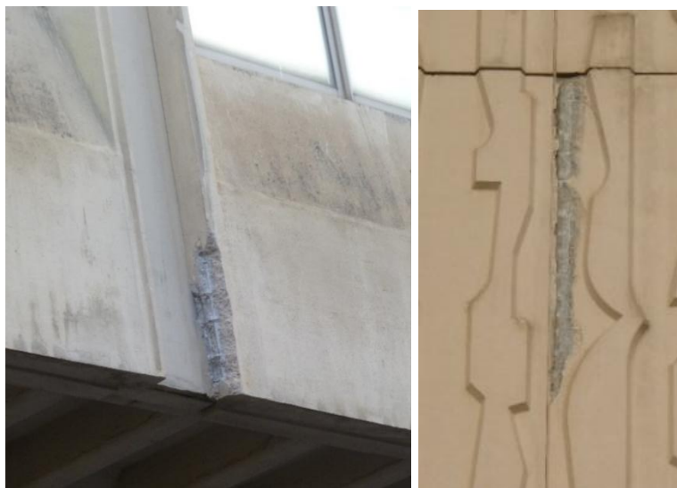
Figure 6.1: Concrete failure is apparent on all facades of the building.
