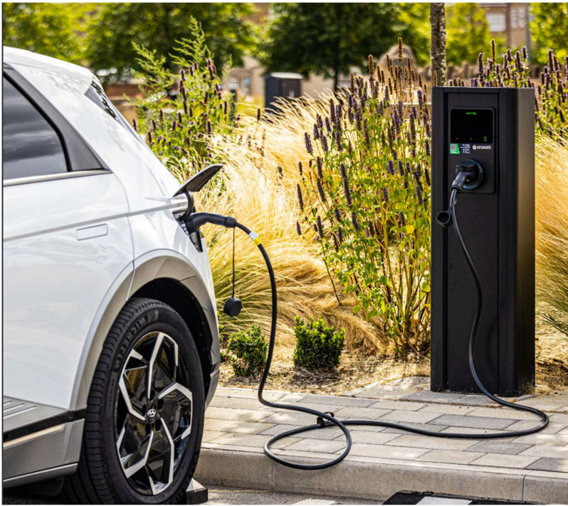
Figure G – Single / Twin pedestal EV Charging points
