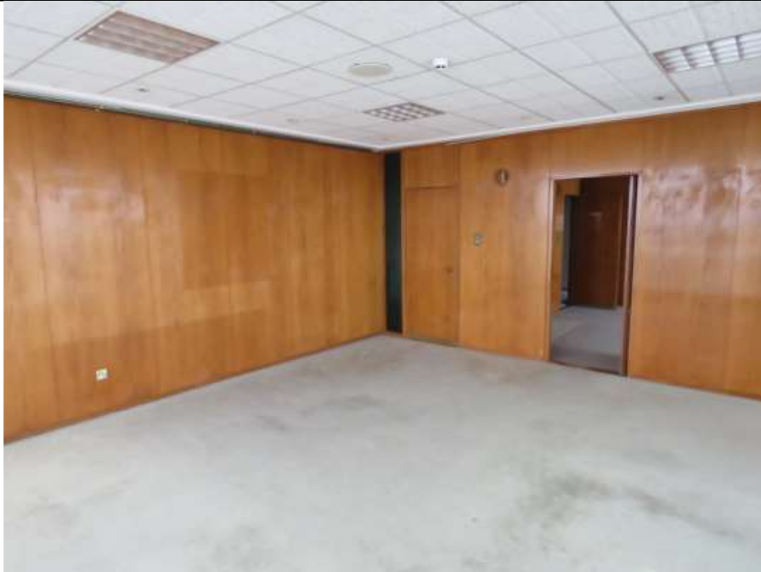
23-16 View south in the General Managers office.
