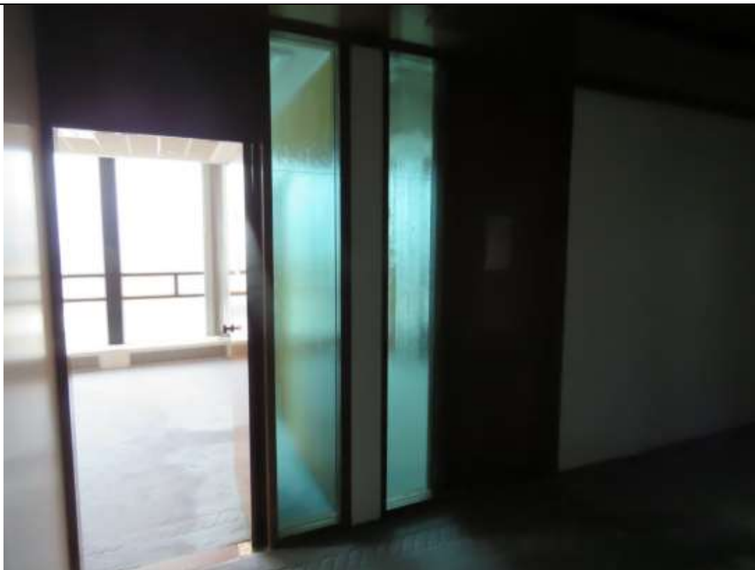
23-11 View of blue obscured glazed panel adjacent to office doors.
