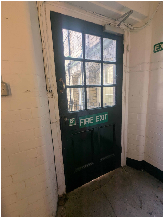
External Escape Door and Internal Details
