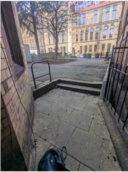
External Escape Door and Escape Route
