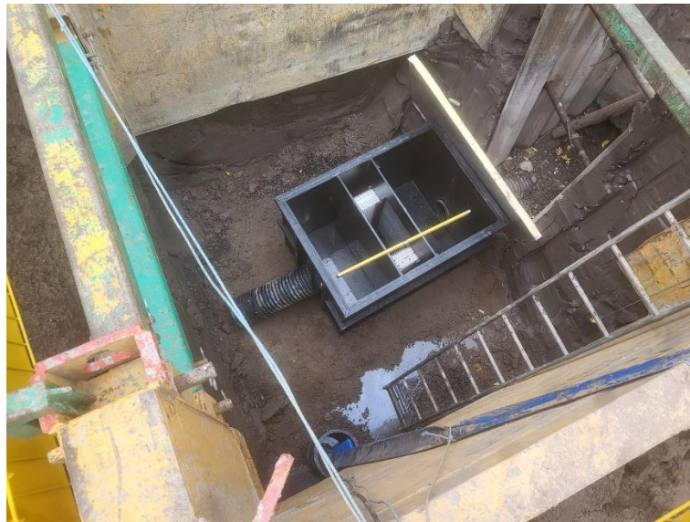
Figure 4 – Smart Filter Chamber
