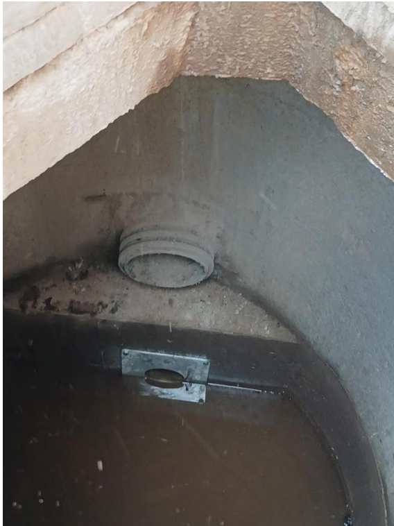
Figure 3 – Flow Control Chamber (Orifice Plate)
