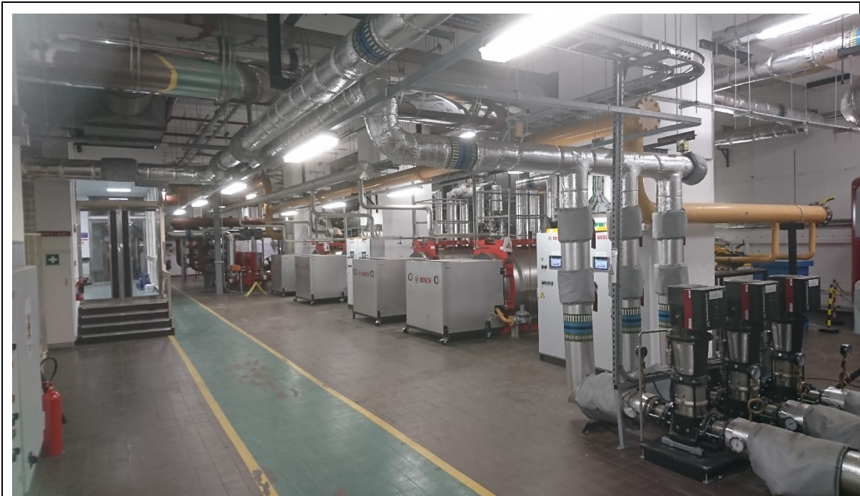
B3-08 Looking north-east to wards ventilation and heating plant, with the control room on the left hand side.
