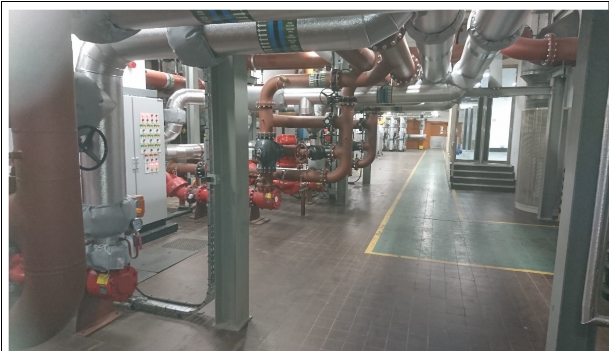
B3-14 View looking south through the main plant room.
