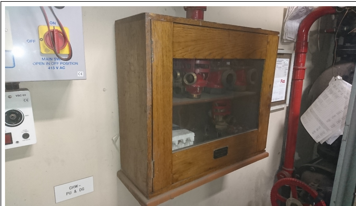
B3-16 View of cabinet with Mulsifyre system components for fire fighting oil fires.
