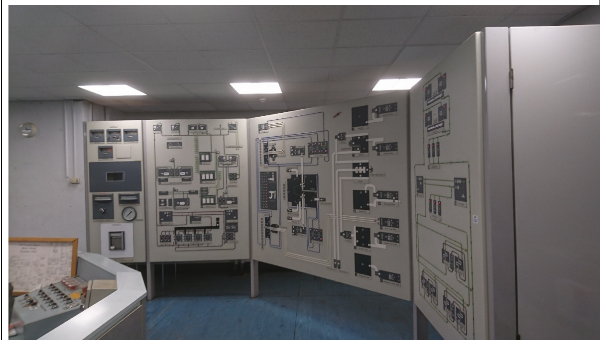
B3-11 The original control panel located within the control room.
