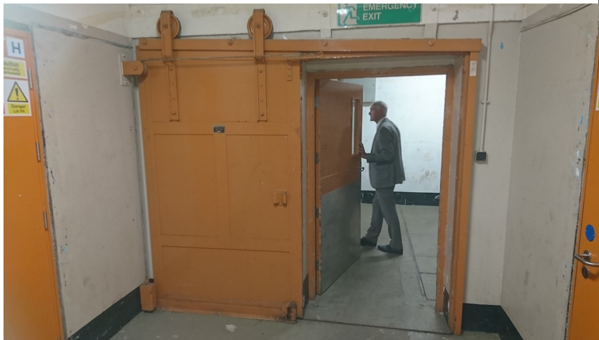
B3-03 View of the fire doors separating the lift core from the basement, which have been upgraded for fire protection and still operational.
