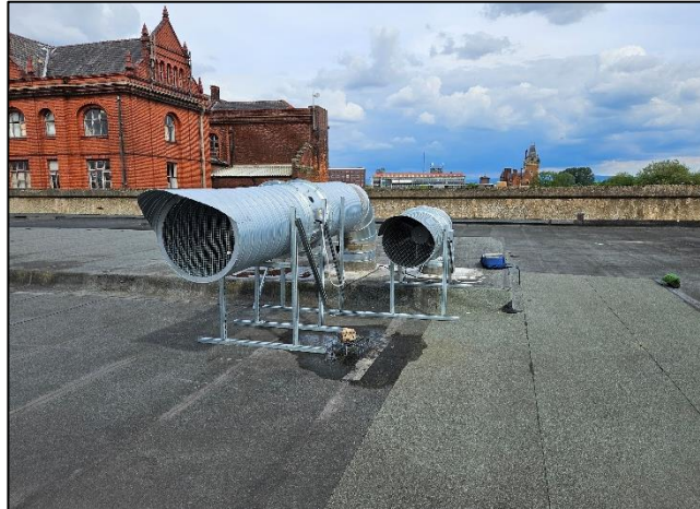
Figure 1 – Roof Top Mounted Supply and Extract Ducts
