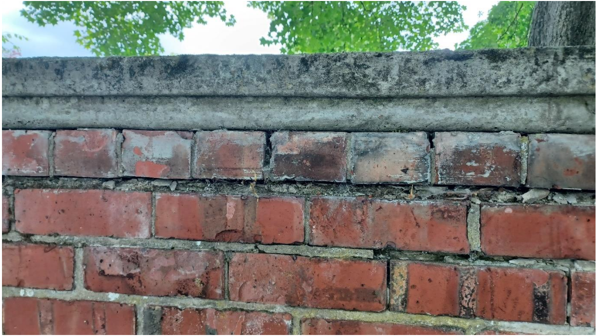
Photo 5: Photograph shows the cast insitu concrete coping on top of the boundary wall and tree roots growing between the brick mortar joints.
