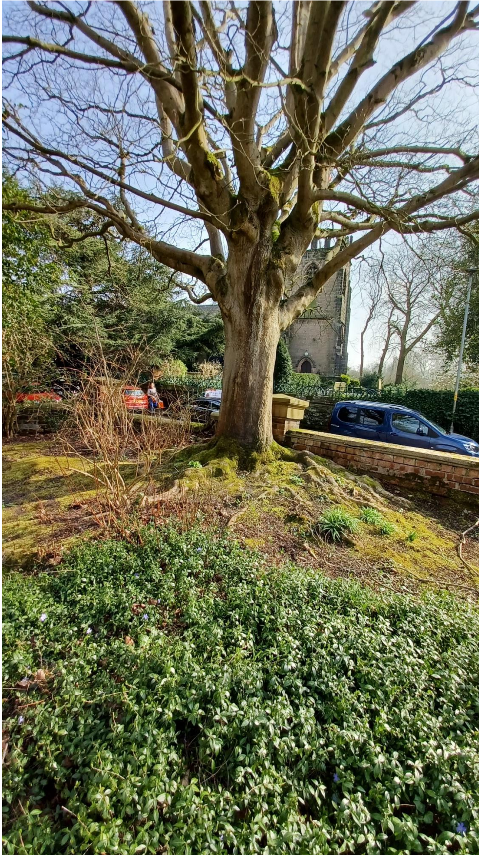
Photo 2: Root system at ground level and parapet wall from inside Parsonage Gardens.
