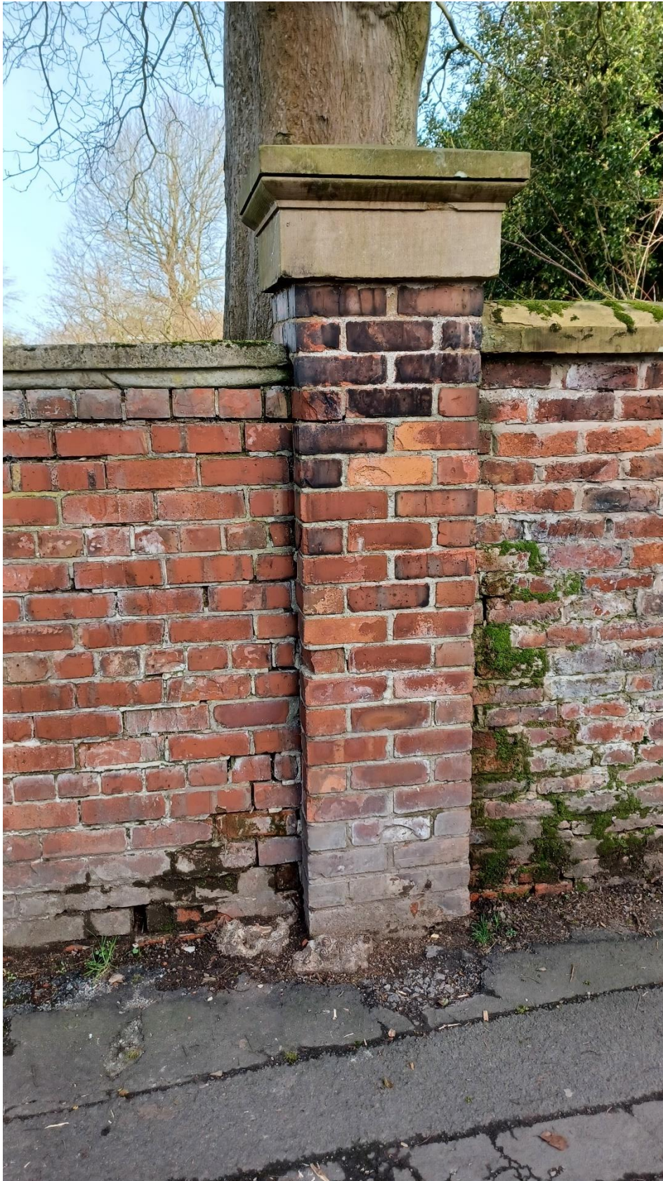
Photo 7: Photograph shows the existing copings, left side newer concrete coping, pier coping and original curved coping on right hand side.
