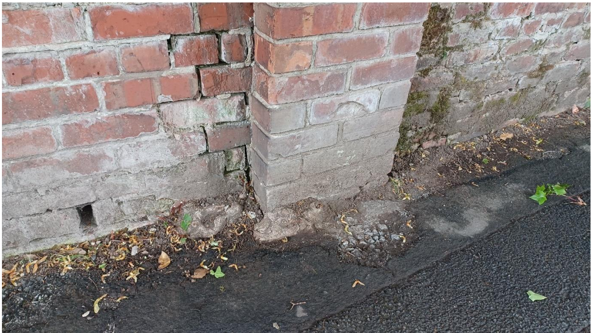
Photo 6: Roots at ground / footpath level at base of pier adjacent Field Maple Tree.
