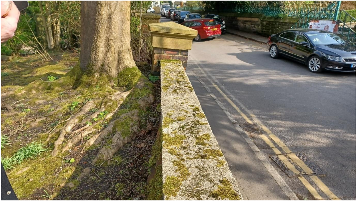
Photo 4: Photograph of the leaning boundary / retaining wall. Photo shows the roots behind the wall are pushing the wall at parapet level.
