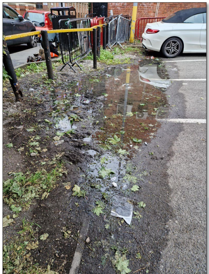
Standing Water In Carpark From FW Gully
