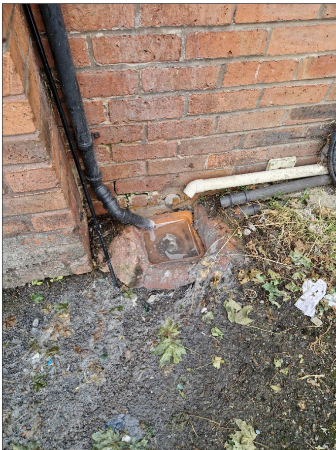
Overflowing FW Gully From Pub
