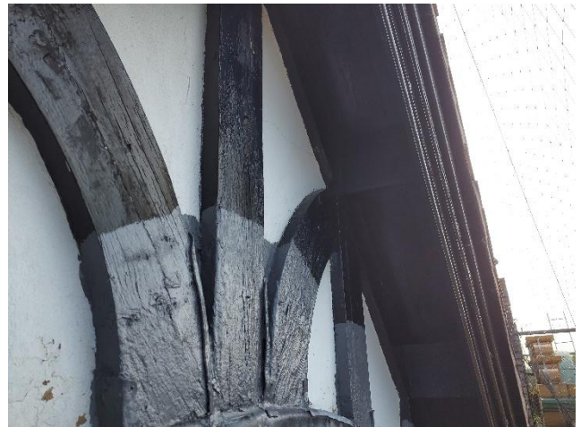
16 Mock tudor timber elements poor condition - Front
