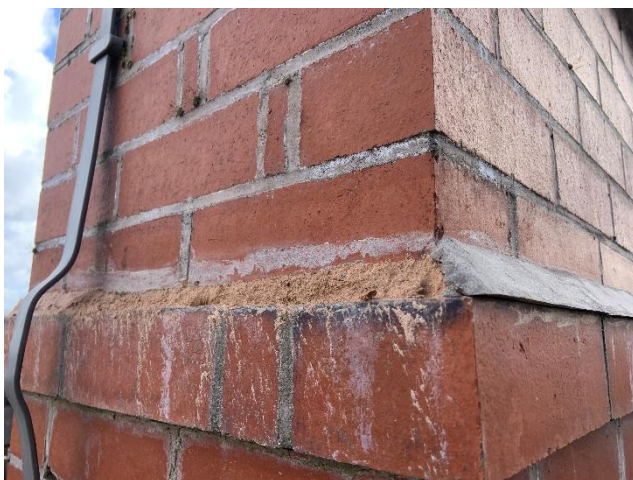
15 Poor pointing repairs to rear chimney
