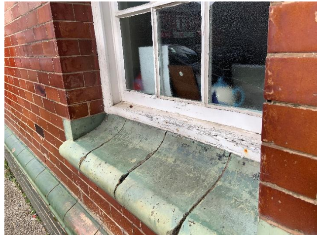
2 round floor windows to be overhauled
