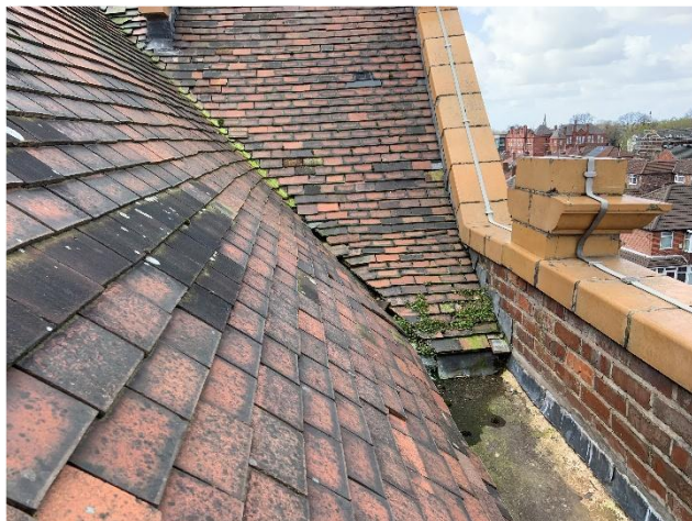
7. Broken and loose tiling to rear pitched roof
