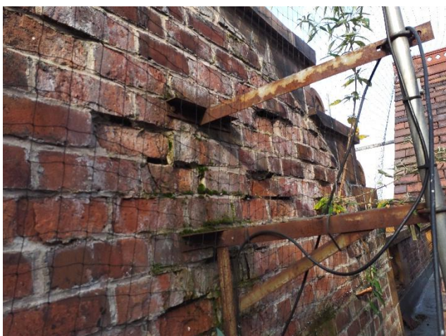
11. Perished brickwork to rear of front pediment
