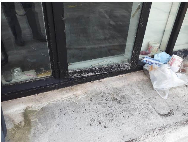
5 Flaking paint to rear dormer windows
