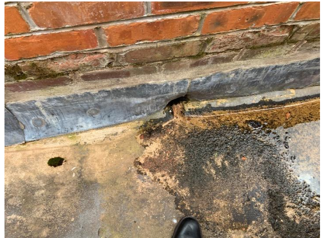
14 Poor drainage to rear flat roof
