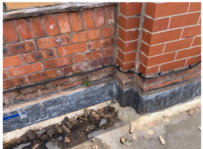
6 Dampness and pointing failing to rear parapet
