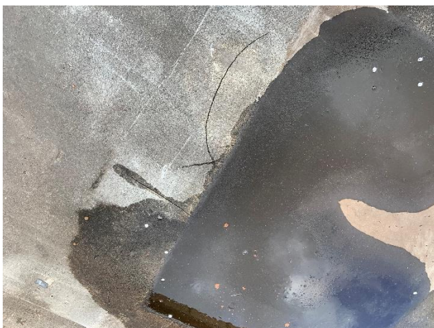
9. Typical cracking to rear asphalt roof covering
