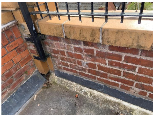
10. Perished brickwork to rear parapet walls
