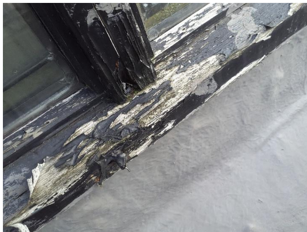
12. Poor condition to front door windows
