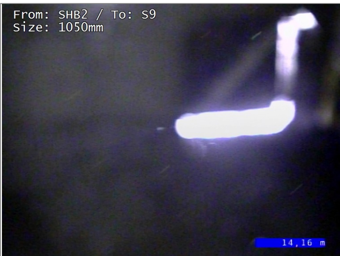
Finish node type, manhole, reference S9
