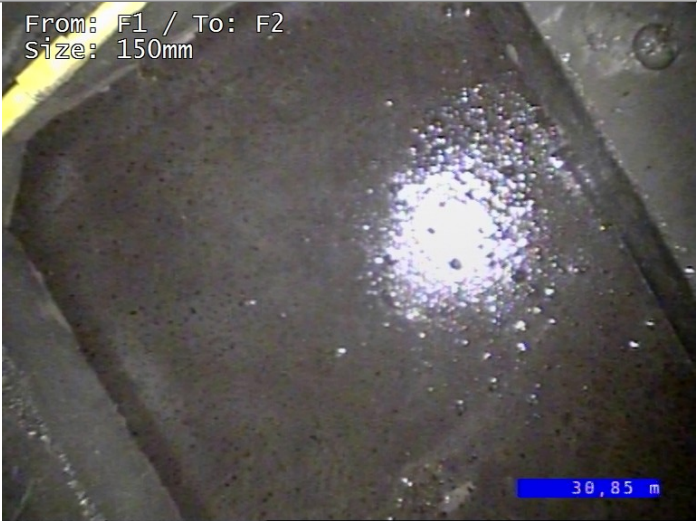
F2, BURIED UNABLE TO FIND
