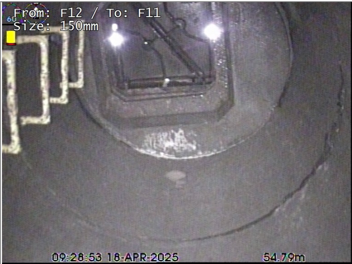
Finish node type, manhole, reference F11
