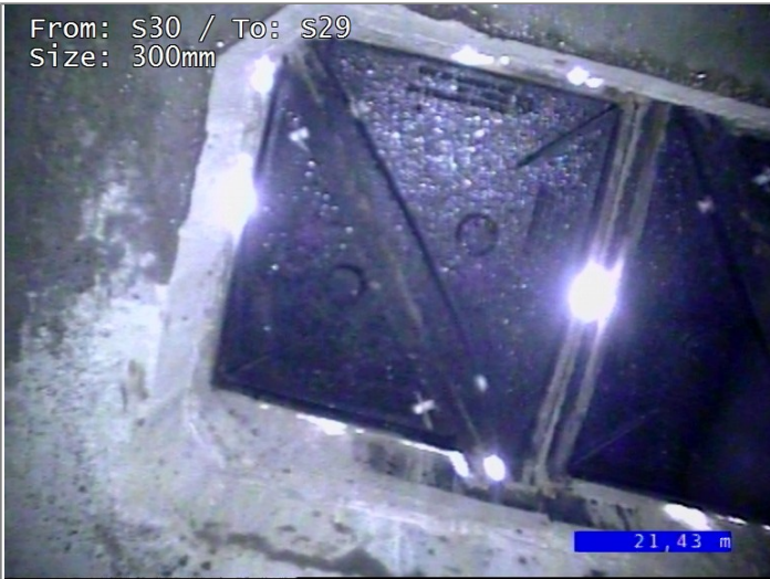
Finish node type, manhole, reference S29
