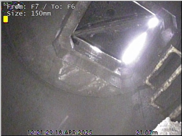
Finish node type, manhole, reference F6
