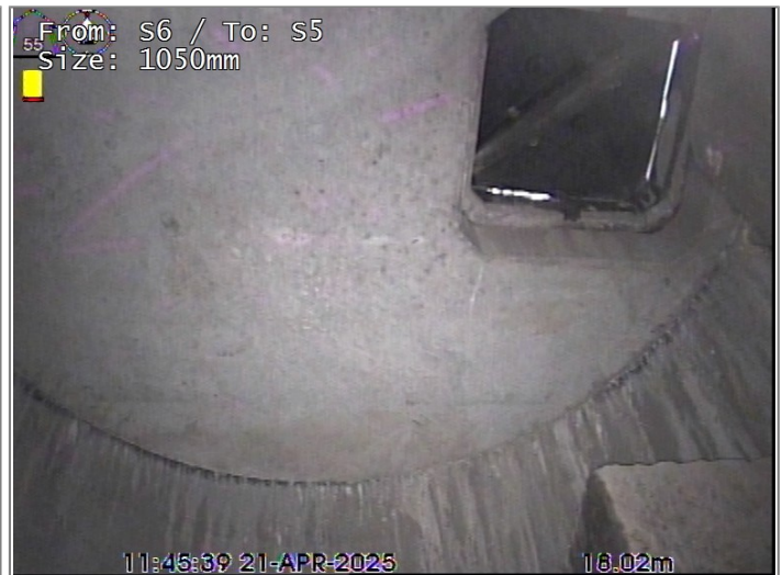
Finish node type, manhole, reference S5
