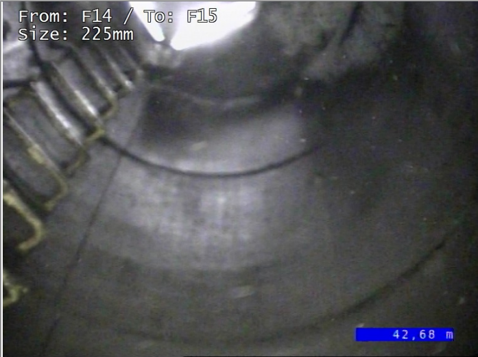
Finish node type, manhole, reference F15
