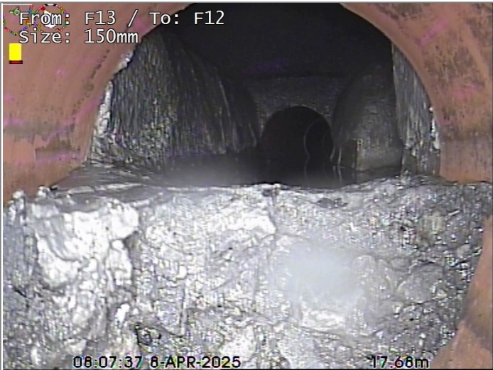
Settled deposits course 50% cross-sectional area loss - Remark: SETTLED CONCRETE
