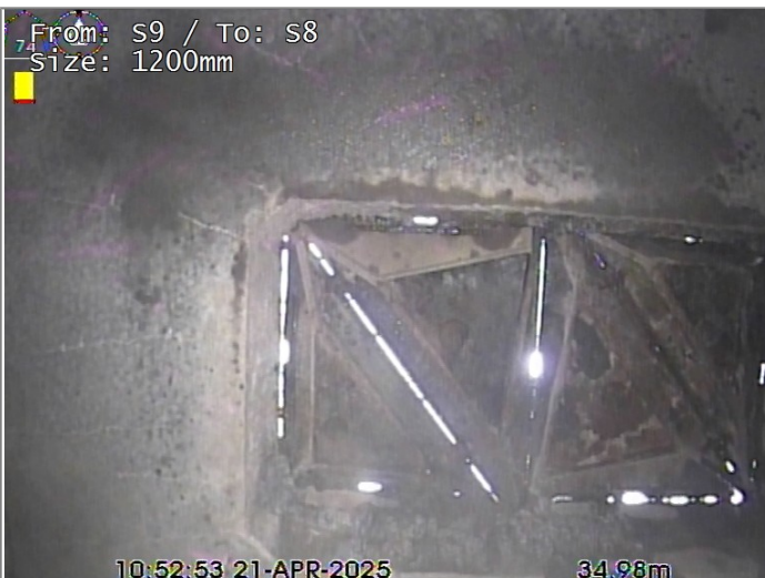
Finish node type, manhole, reference S8
