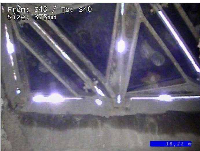
Finish node type, manhole, reference S40
