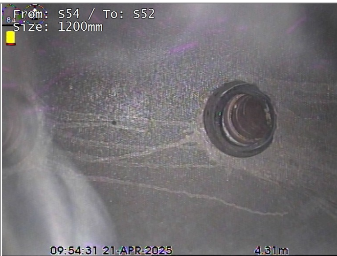
Connection other than junction at 2 o'clock, diameter 150mm
