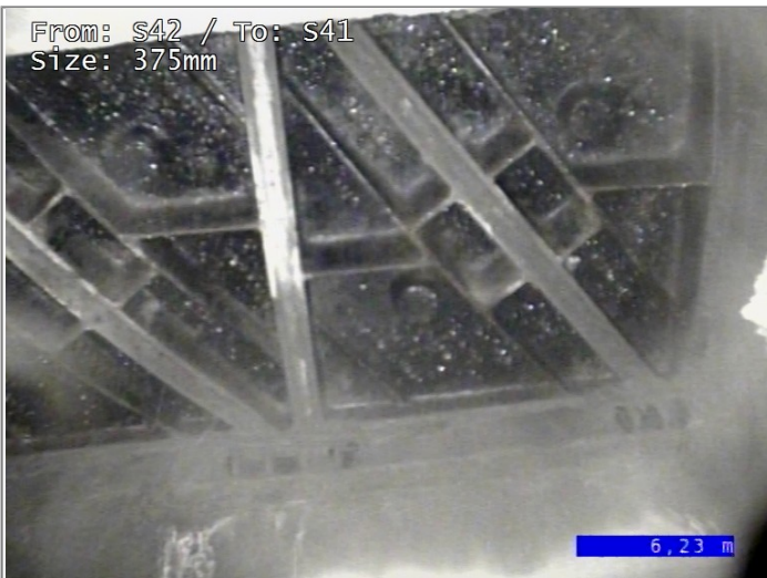
Finish node type, manhole, reference S41
