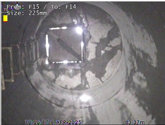
Finish node type, manhole, reference F14
