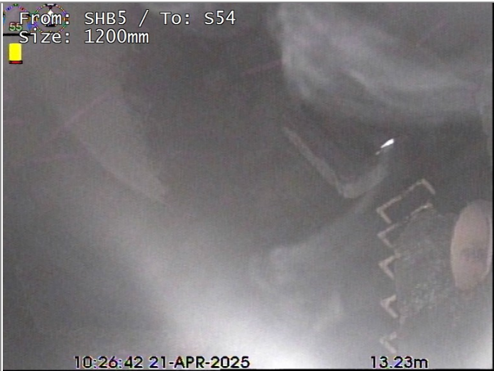
Finish node type, manhole, reference S54
