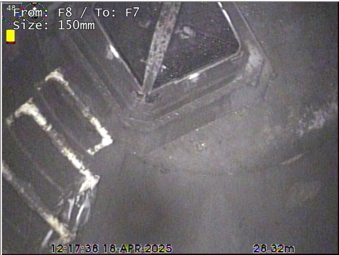
Finish node type, manhole, reference F7
