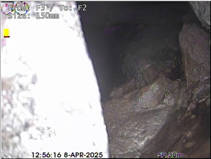
Finish node type, manhole, reference F2
