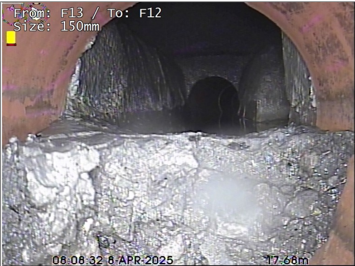
Survey abandoned - Remark: DUE TO CONCRETE
