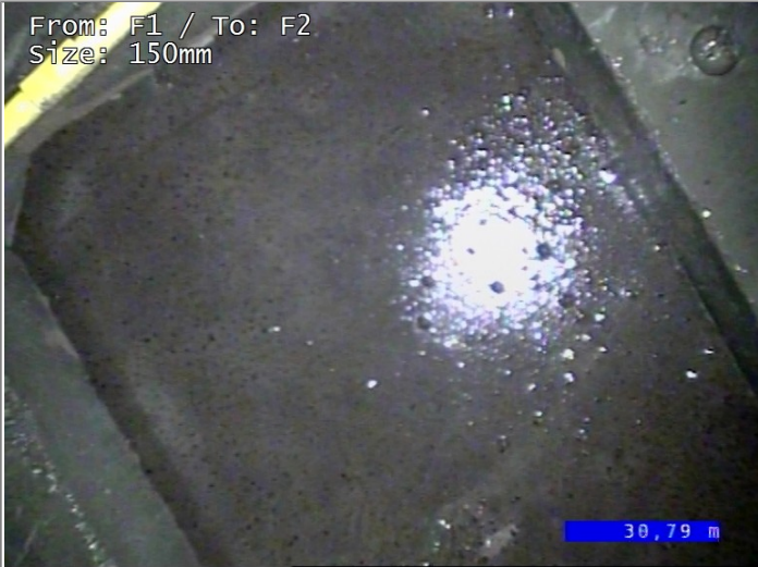
Finish node type, manhole, reference F2
