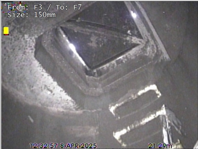
Finish node type, manhole, reference F7
