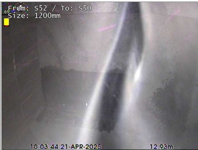
Finish node type, manhole, reference S50
