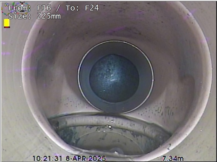
Finish node type, manhole, reference F24
