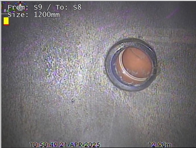
Connection other than junction at 2 o'clock, diameter 150mm
