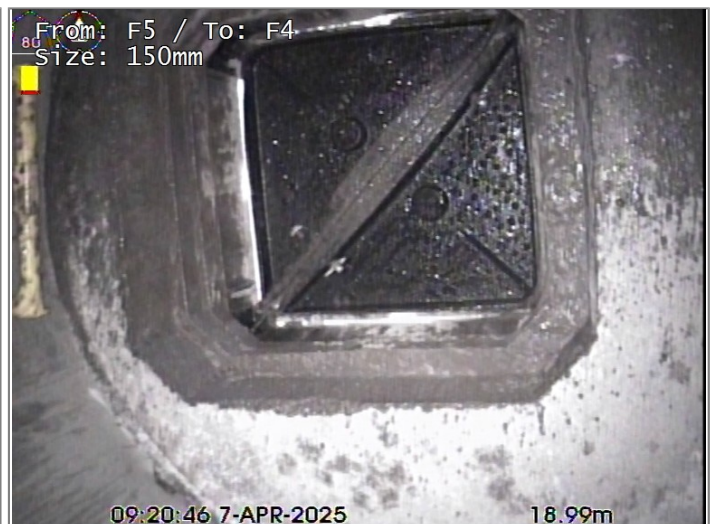
Finish node type, manhole, reference F4
