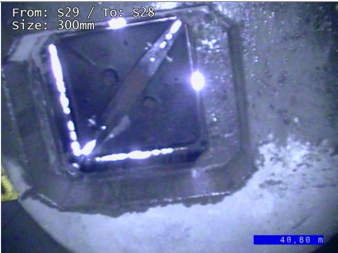
Finish node type, manhole, reference S28
