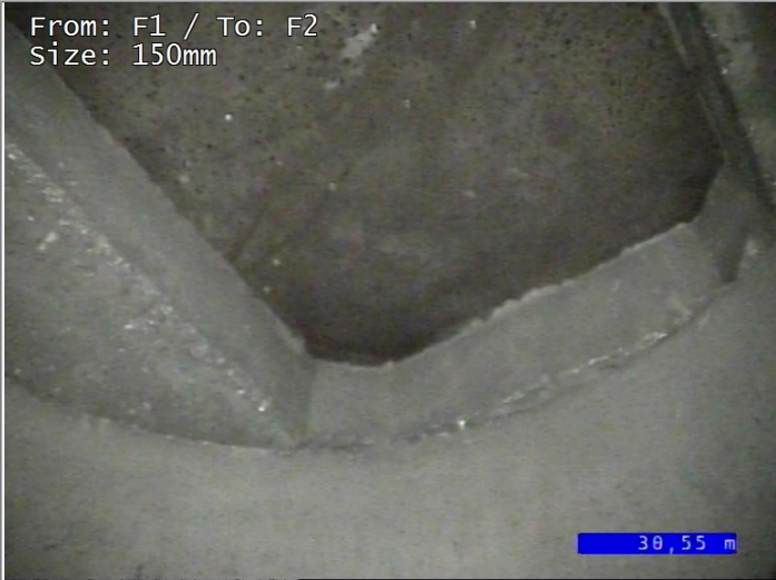
Finish node type, manhole, reference F2
