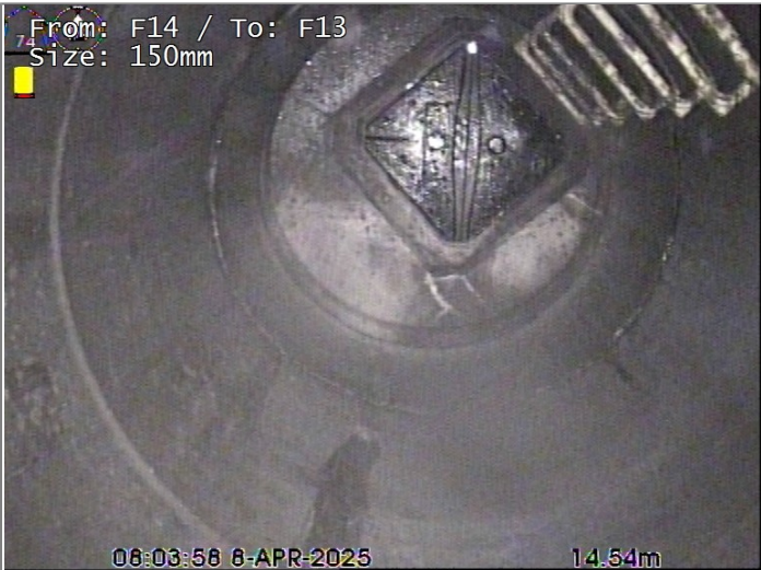
Finish node type, manhole, reference F13
