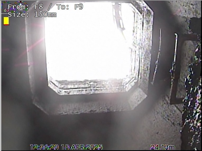
Finish node type, manhole, reference F9
