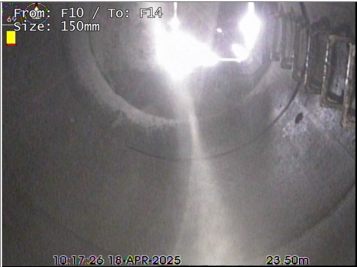
Finish node type, manhole, reference F14
