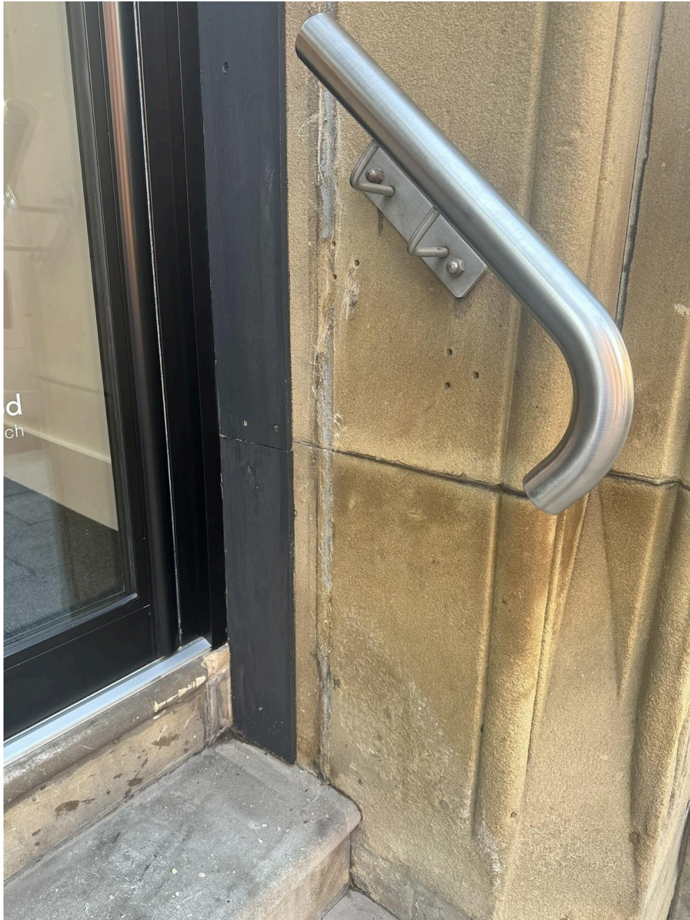
Figure 4.0 - Old handrail fixing holes
