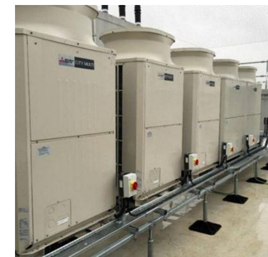
Figure 10 - Typical External Condenser
