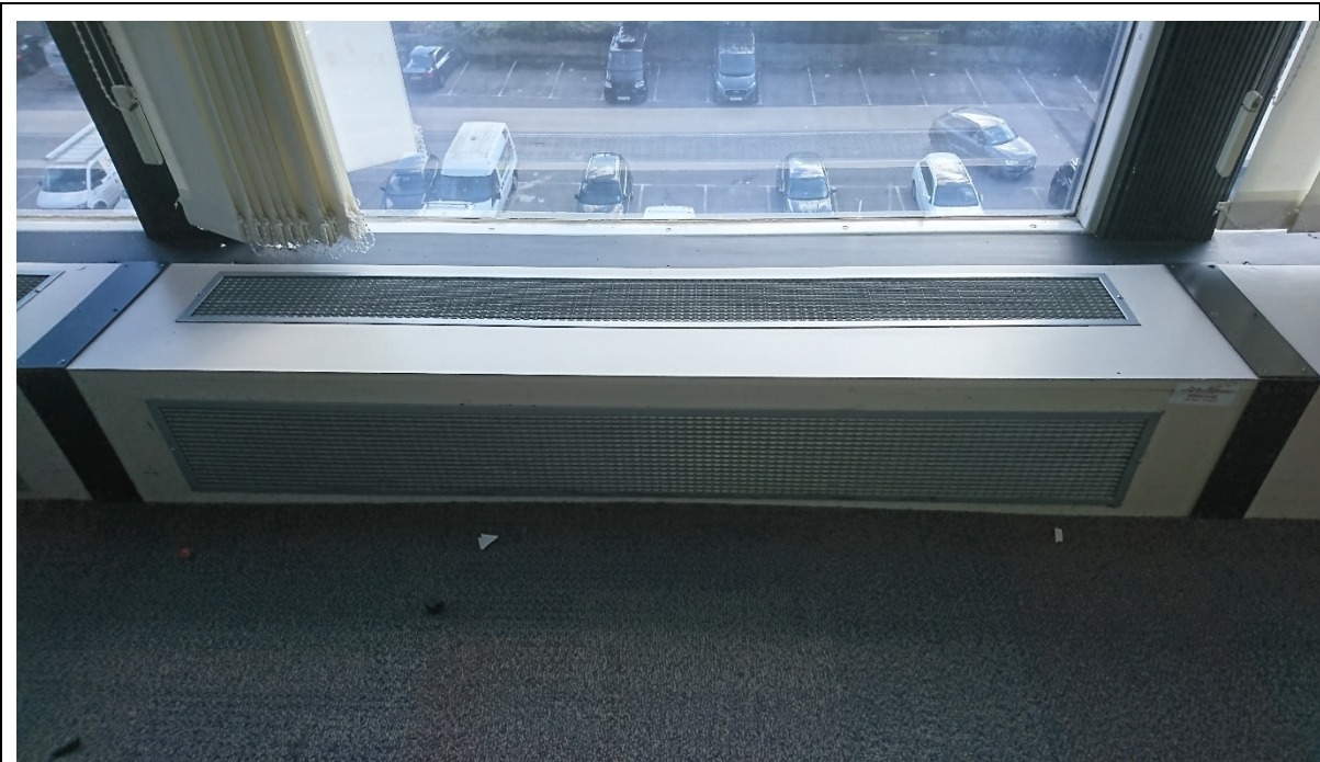
04-22 Weathermaster conduit and vent grills to the perimeter of the floor.
