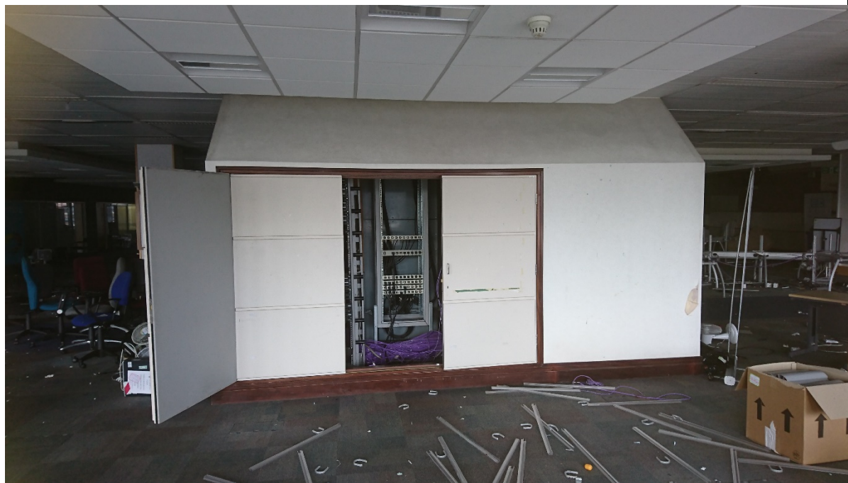
04-23 View of service cupboard with IT racking and cabling.
