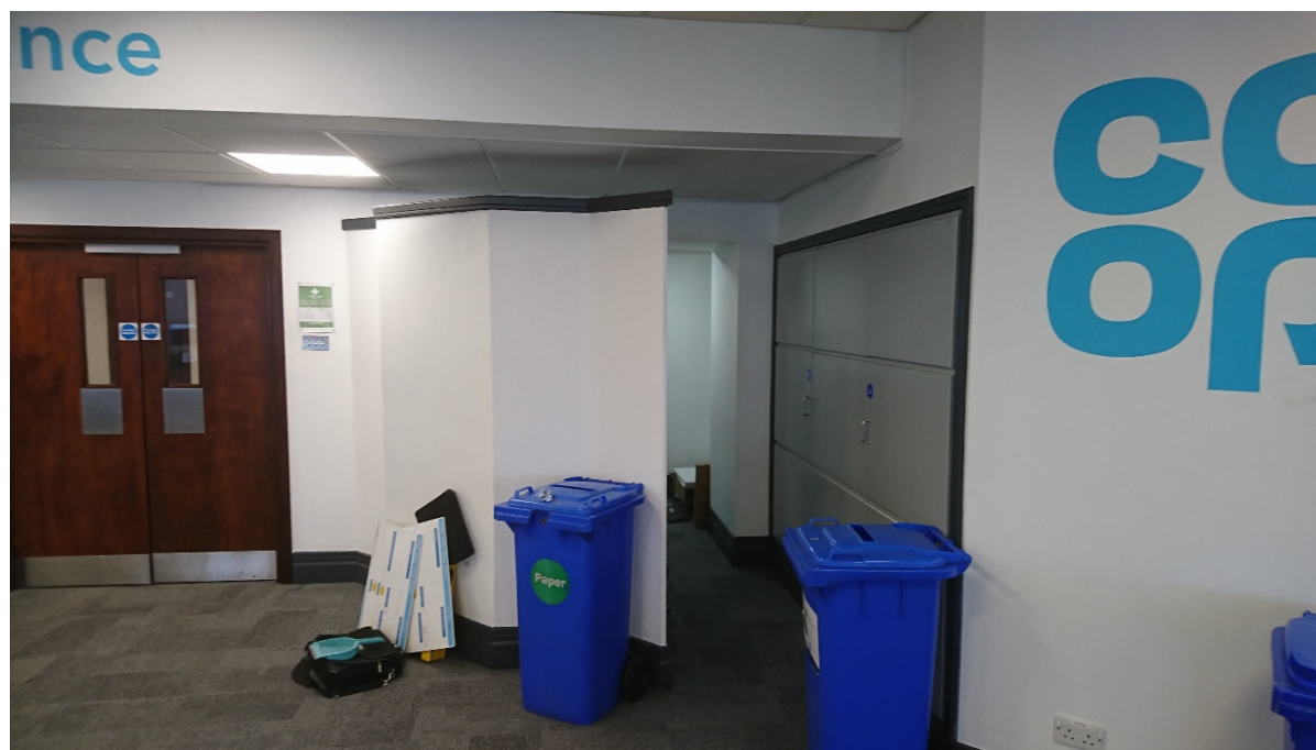
04-05 The internal screen of the telelift system adjacent to the lift lobby.
