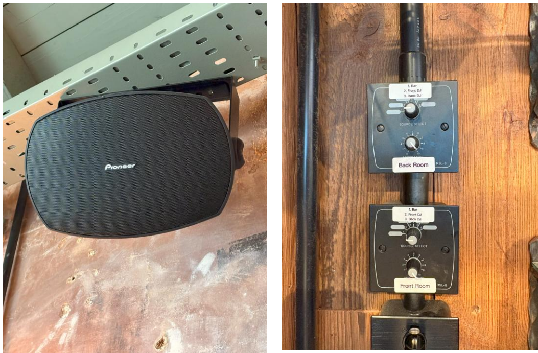
Figure 4 Photograph of loudspeaker and controller unit
