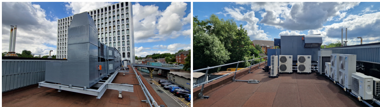
Images 1 and 2: Newly Installed AHU Plant And External Air To Water Heat Pumps
