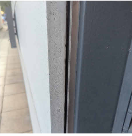
Existing Flashings and Cills
