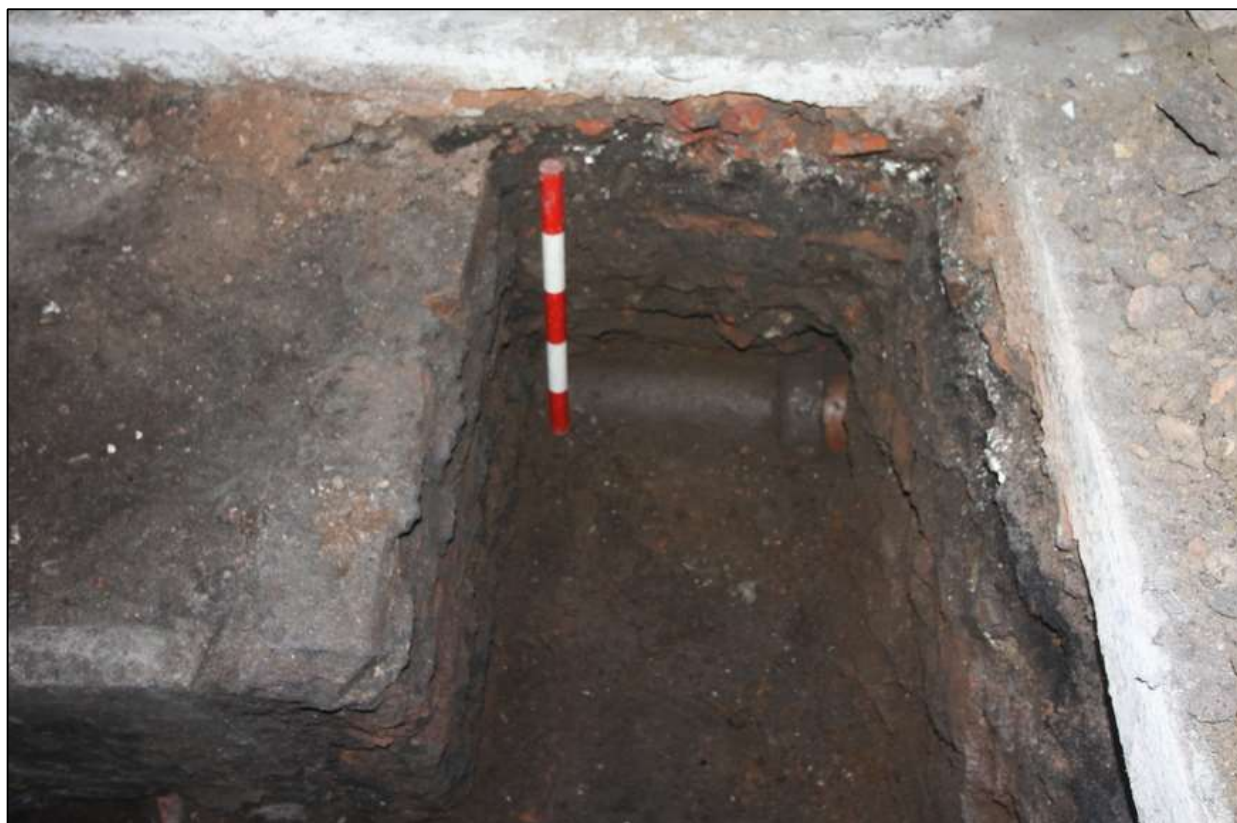
Plate 70: Salt-glazed ceramic drainage pipe revealed in the western section of the test pit
