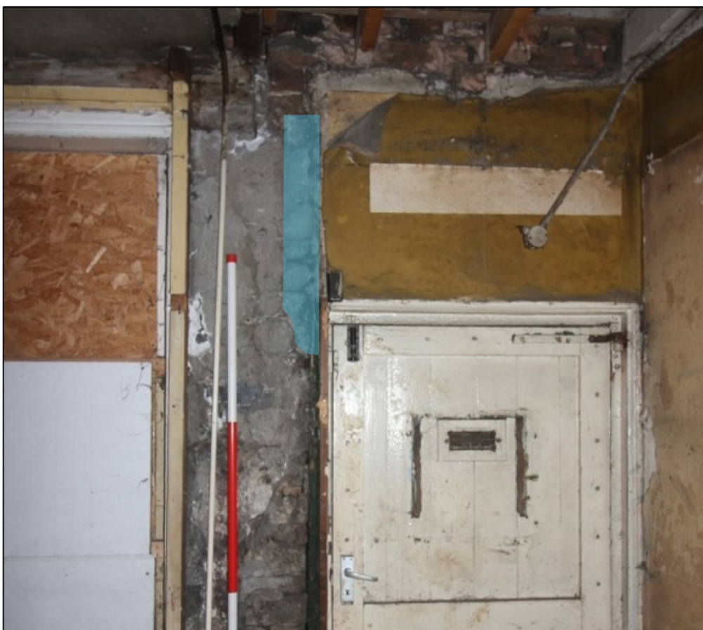
Plate 34: Slight wall scar for probably partition wall of ground-floor level corridor from entrance door
