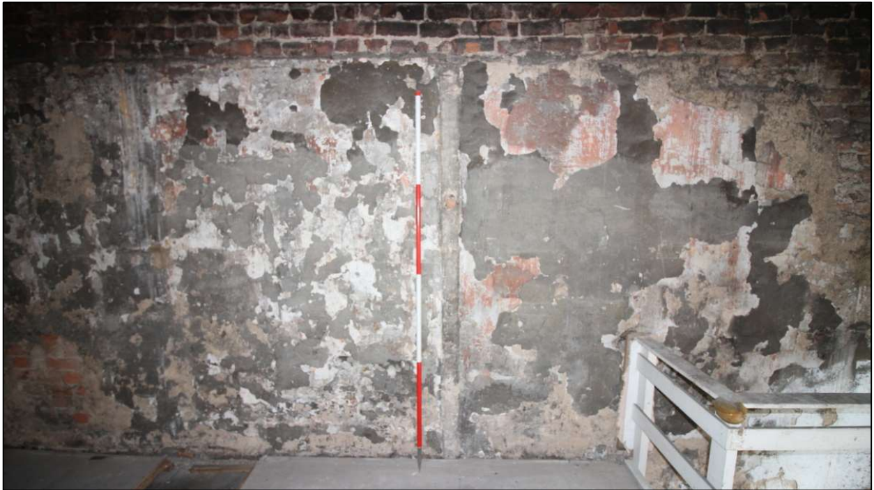
Plate 60: East wall of upper floor, with vertical scar for single-skin brick partition wall
