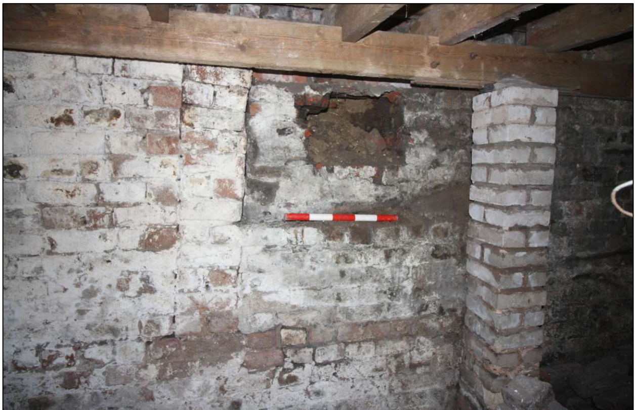
Plate 42: Blocked cellar light window in rear wall of cellar
