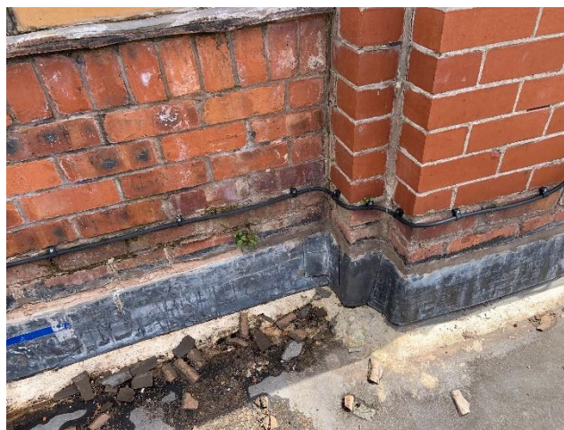
View of rear parapet wall and loose flashings.
