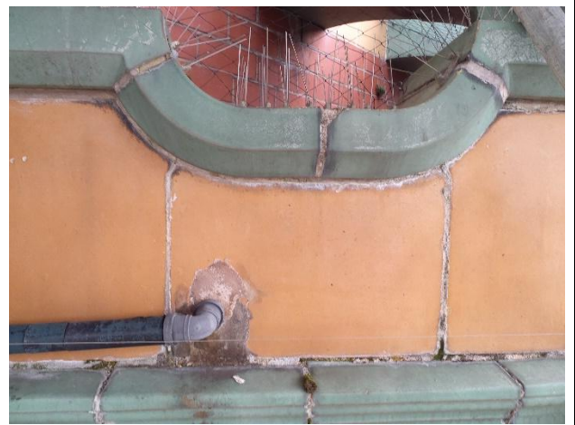
Image 74: Staining around bay roof drainage pipe.
