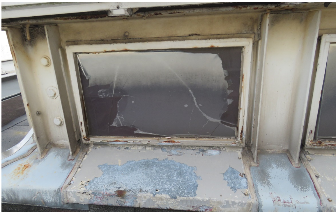
RL 05 Detail of the original upstand and clerestory glazing of the pyramid roof, showing the failing, applied protective film.
