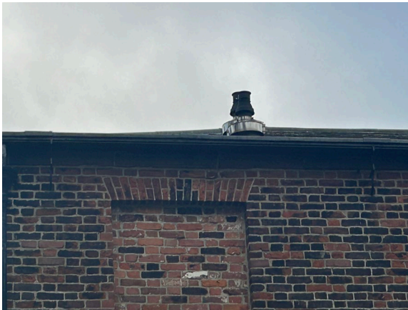
Boiler Flues Penetrating Roof
