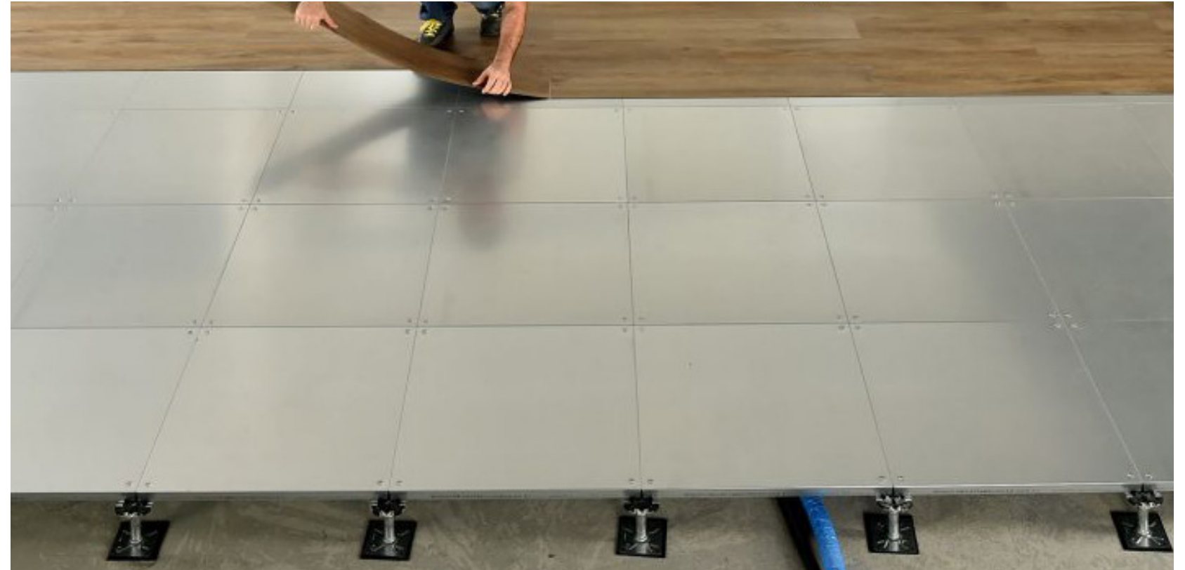
RAISED ACCESS FLOOR
