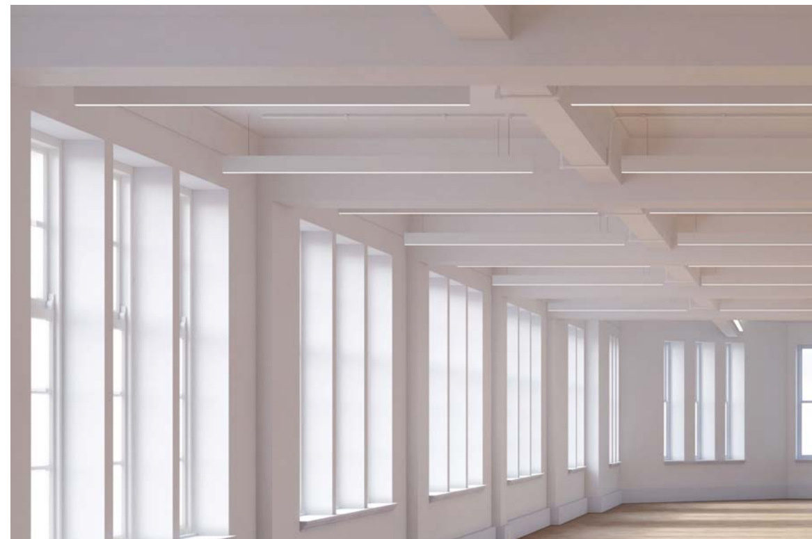
New linear lighting inbetween the cofferes
