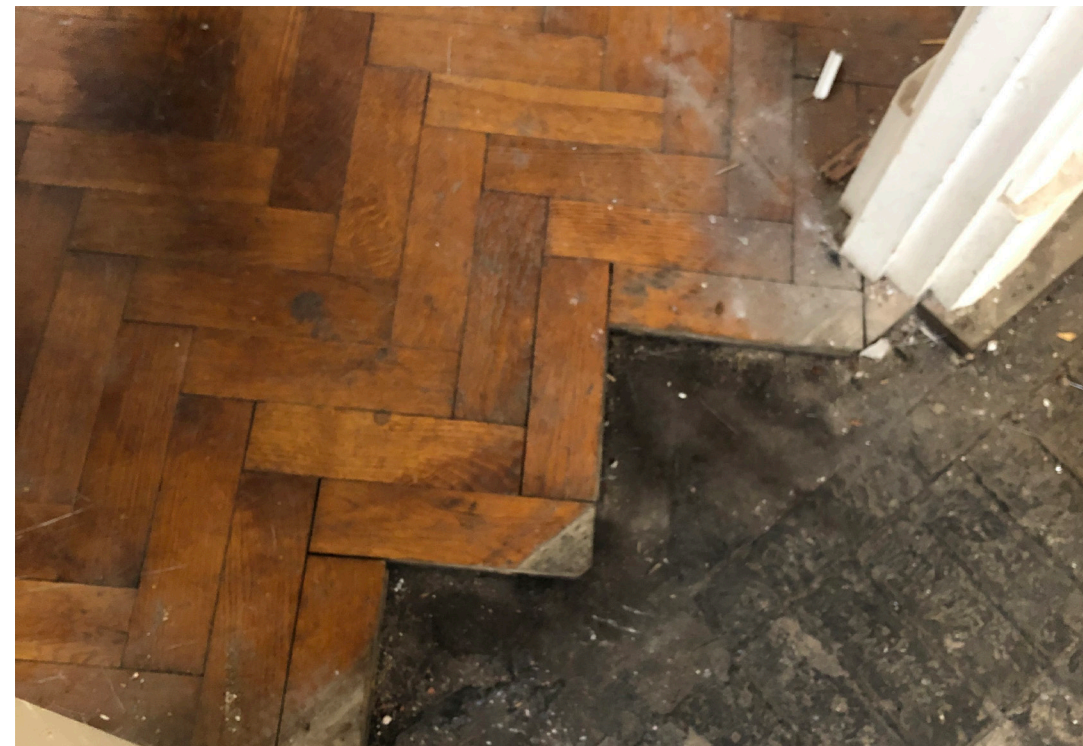
B. INFIL TO PARQUET FLOORING IN PLACES
