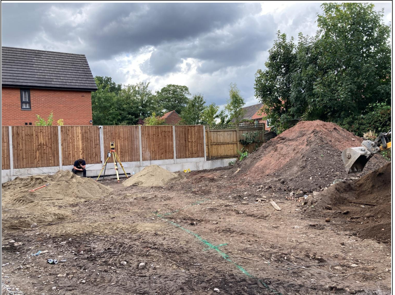
Figure 5: Back garden area, showing 600 mm strip has not be completed to date. Facing northwest.
