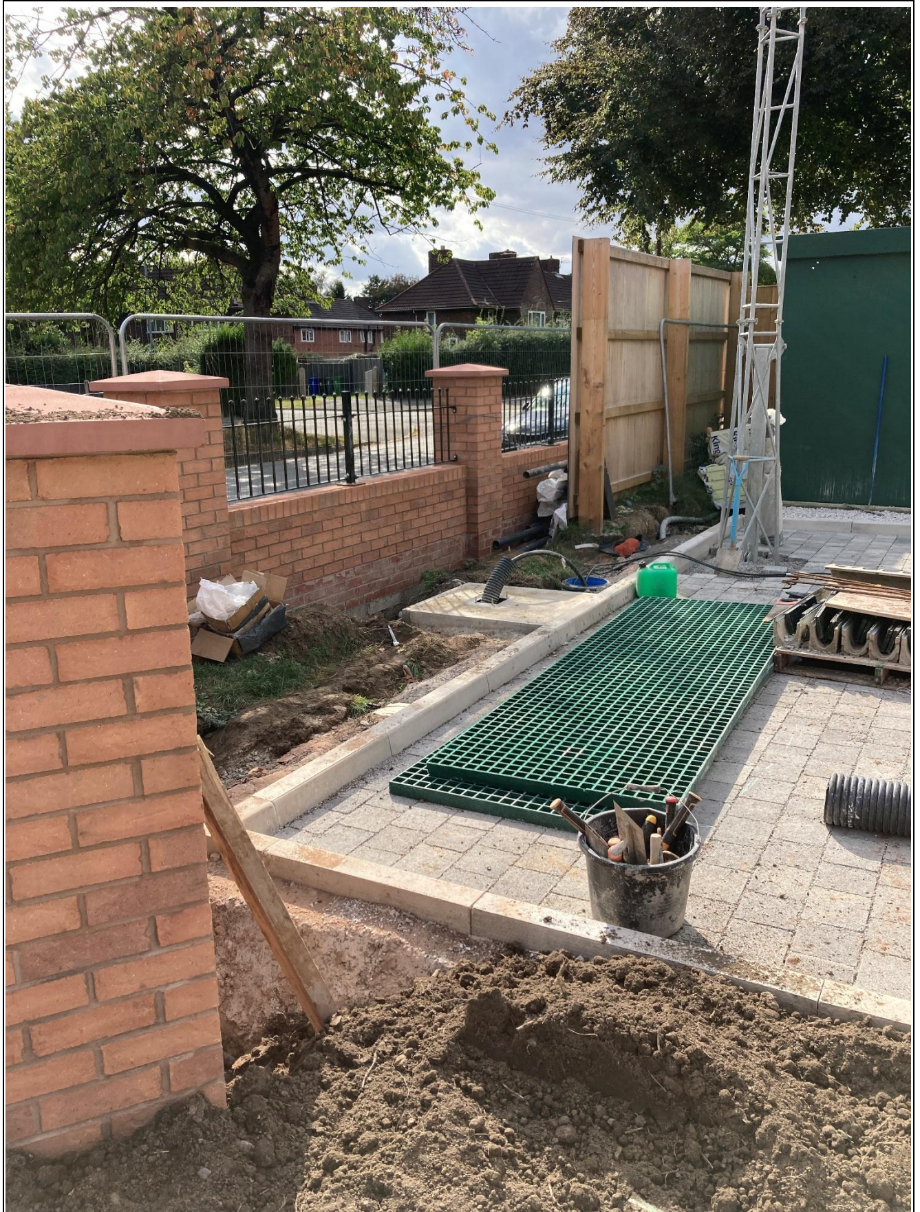
Figure 3: Southwestern corner of the car park, showing incomplete clean cover system. 600 mm strip and installation of system needed needed in this bed. Facing southwest.
