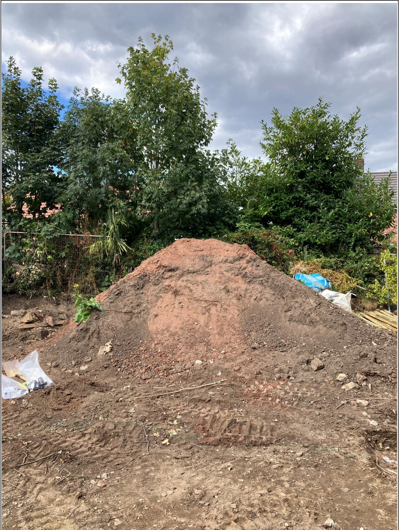
Figure 6: Photograph of SP01, imported for use within the clean cover system in the back garden. Facing north.
