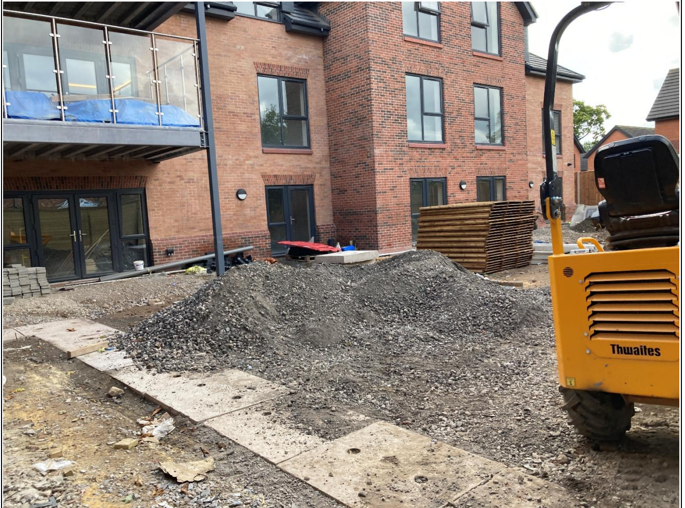
Figure 4: Back garden area, showing 600 mm strip has not be completed to date. Facing southwest.
