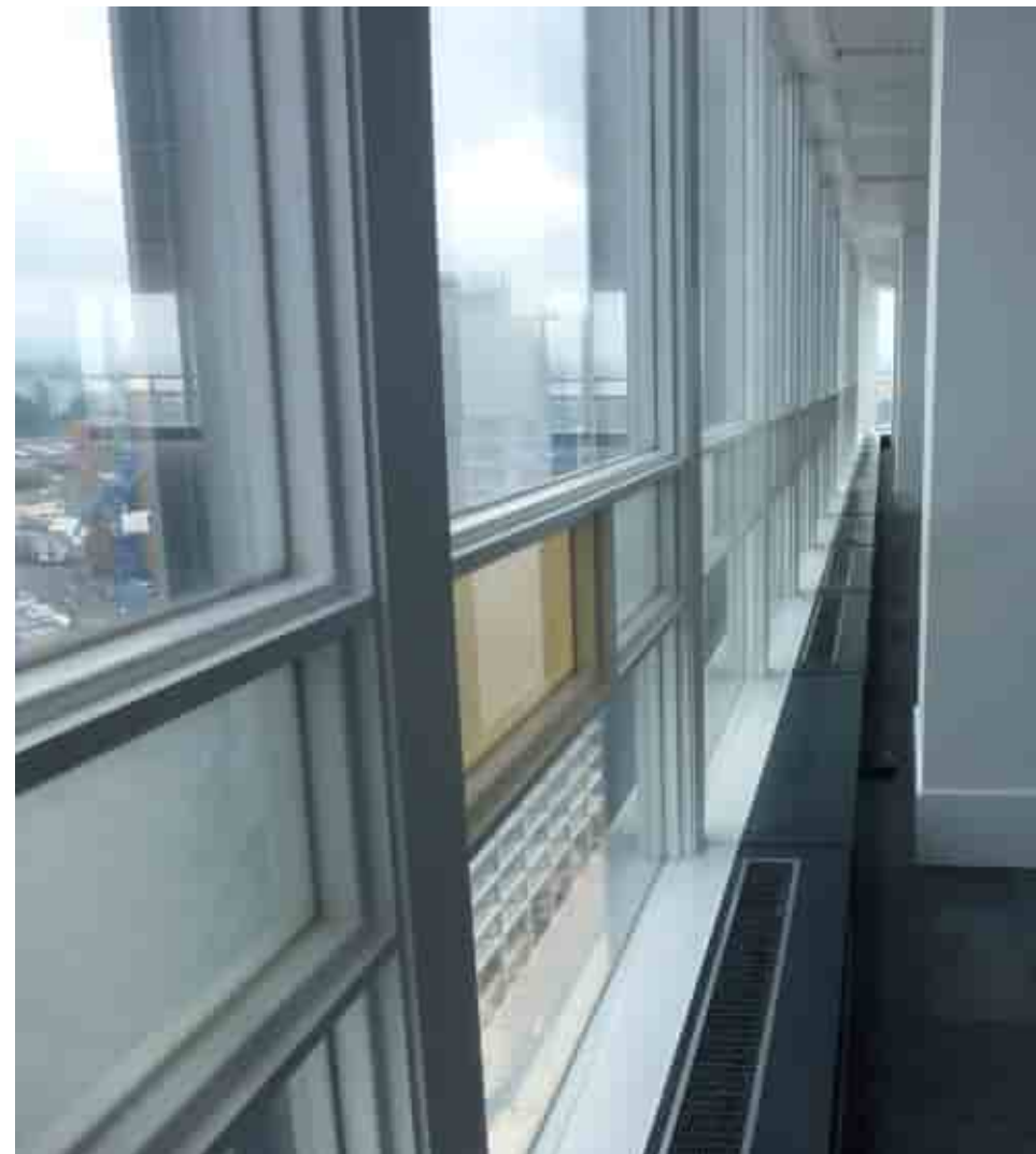
Existing Weathermaster containment
