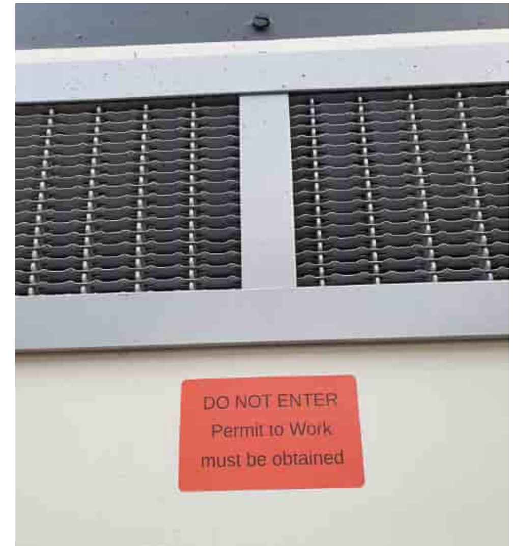
Warning signage placed on containment
