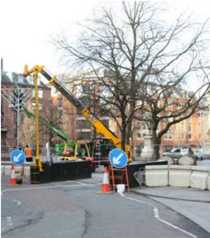
HVM (Hostile Vehicle Mitigation) barrier to Albert Square
