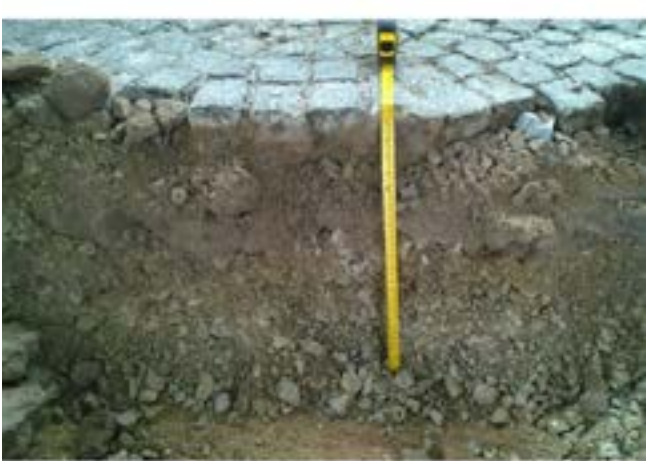
Intrusive survey photos showing extent of roots
