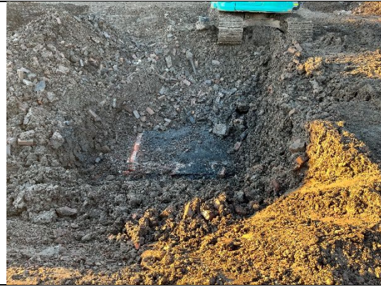
Photograph 6: Hydrocarbon staining on the concrete slab in the northern side of Area 2.
