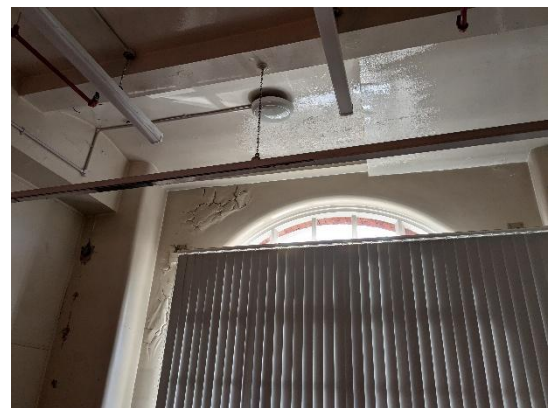
Figure 23: Inappropriate blind and servicing extrusions in office/store (GF.09) in centre of ground floor plan.
