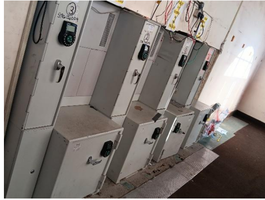
Figure 15: Cash drop machines, to be relocated and re-used, Money Drop Office (GF.07).
