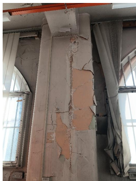
Figure 13: Evidence of historic damp and damage to plaster work in Money Drop Office (GF.07).
