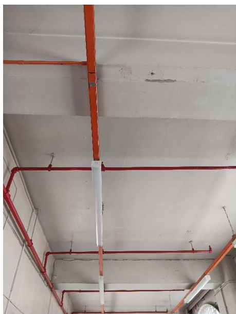
Figure 12: Historic sprinkler system in Money Drop Office (GF.07), assumed altered to adjust to partition insertion in c.1950s.
