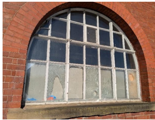
Figure 9: Damage to round-headed window on Queens Road frontage.
