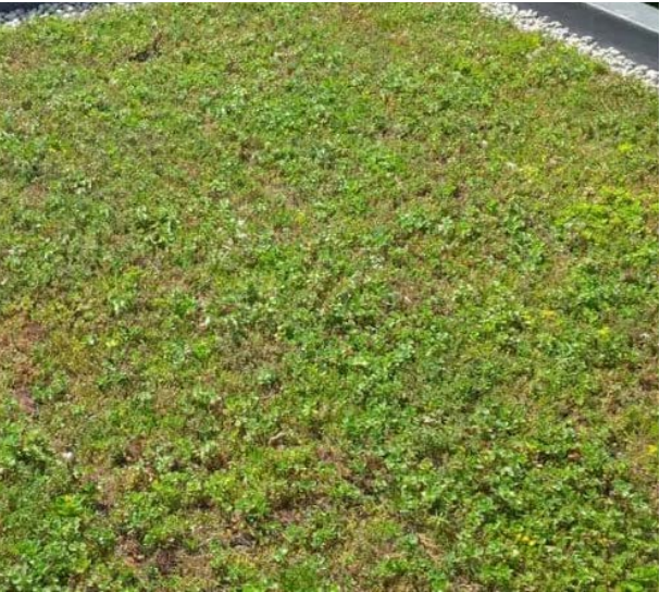
Roof - Green Bauder Matting
