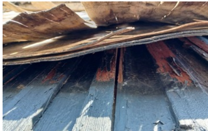
Image 10: Lifted wooden panelling along the external elevation of B1
