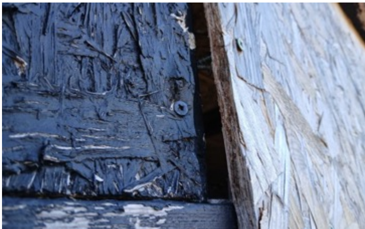
Image 9: Gap present between the wooden panelling on B1
