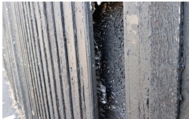
Image 12: Lifted external panelling along B1
