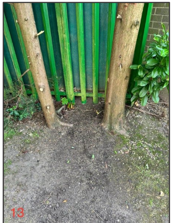
Picture 12. Root severance evident for 2 trees in H13# for cable installation.
