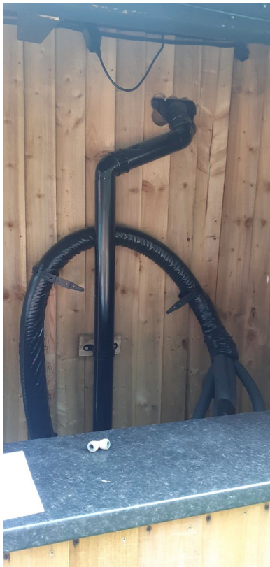
RWP discharging main roof collector pipe through decking boards
