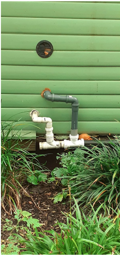
External drainage from kitchen
