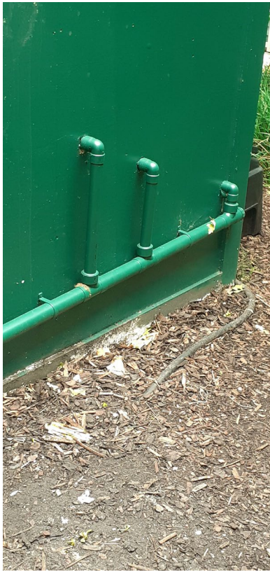
External drainage from kitchen
