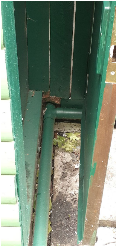
External drainage re-entering building
