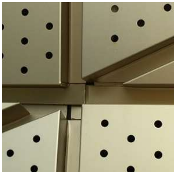
Figure 1 Rainscreen panel corner quality. Aesthetic Reference, Central Bank, Dublin
