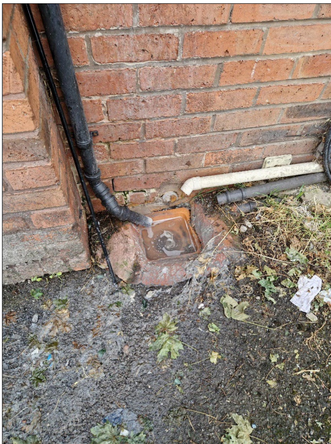
Overflowing FW Gully From Pub
