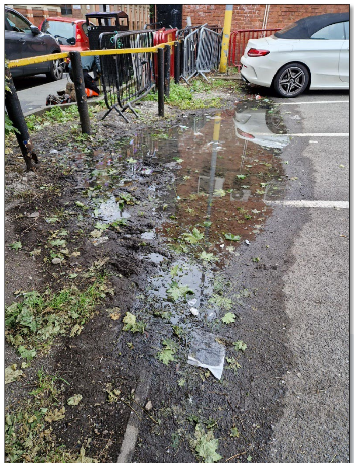
Standing Water In Carpark From FW Gully
